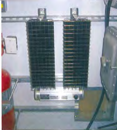
Electrical room heaters
