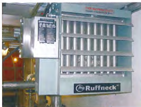
Fueling area heater
