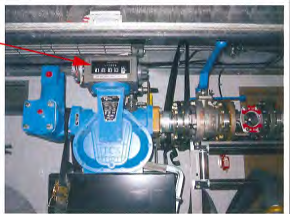
Tanker truck fuel meter
