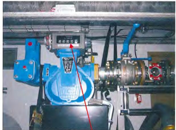
Tanker truck fuel meter
