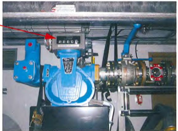
Tanker truck fuel meter
