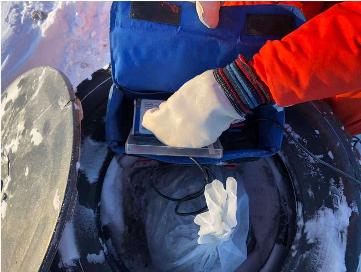
Figure 3 – Blast Monitoring Station installed directly on the ground
