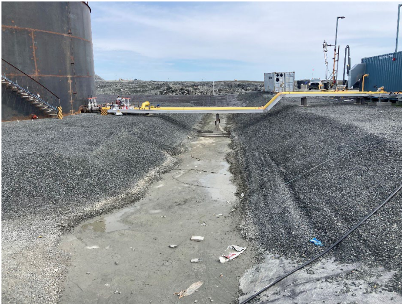
Photograph G3-06 Whale Tail Project Site Tank Farm
