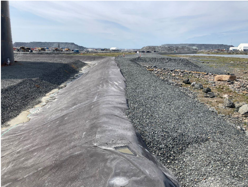
Photograph G3-03 Whale Tail Project Site Tank Farm
