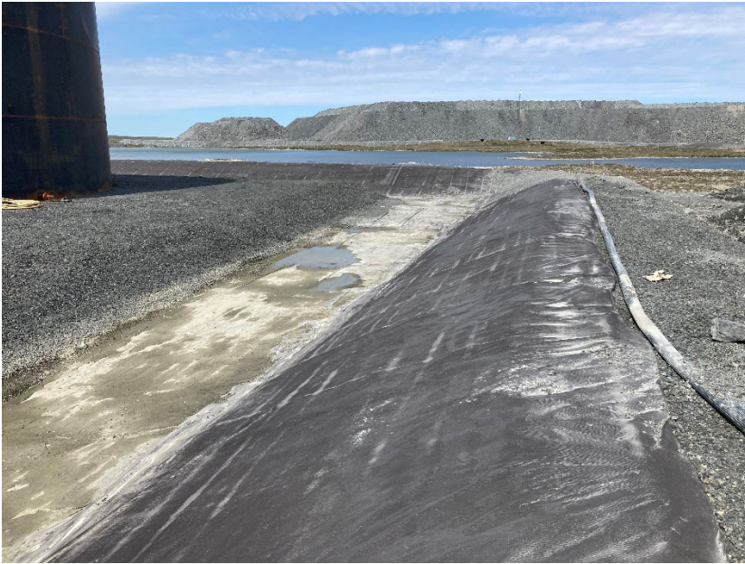
Photograph G3-01 Whale Tail Project Site Tank Farm
