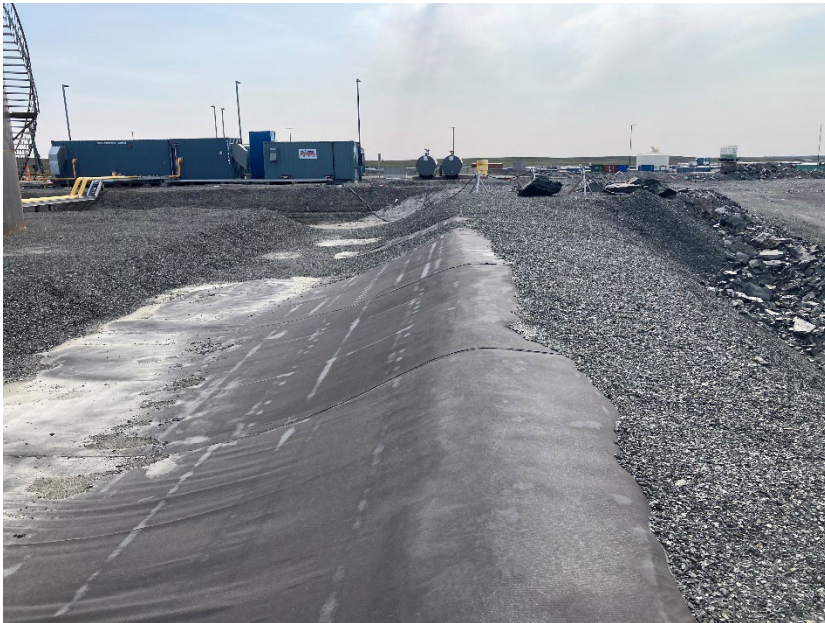
Photograph G3-04 Whale Tail Project Site Tank Farm
