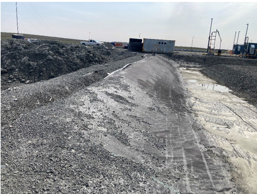
Photograph G3-02 Whale Tail Project Site Tank Farm
