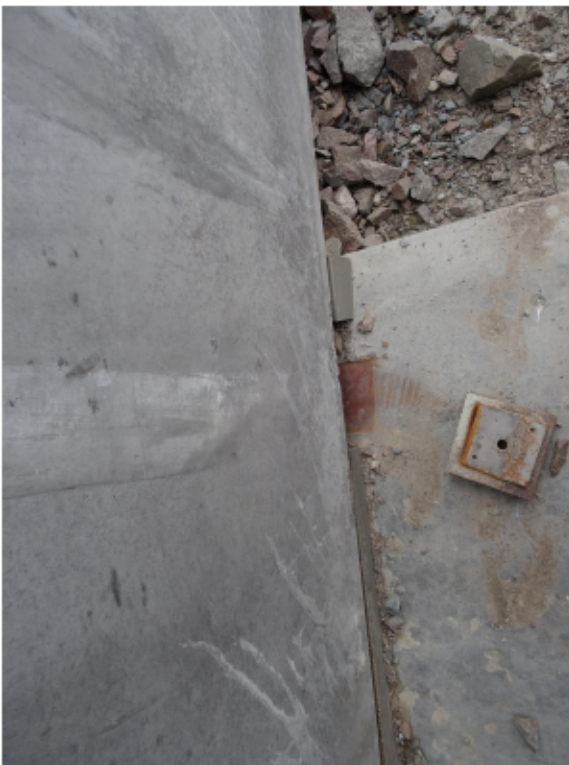
Figure 17: Base of ballast wall - evazote gaps observed (NE)
