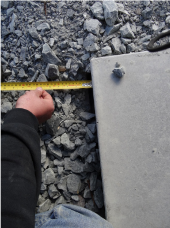
Figure 10: NW footing movement
