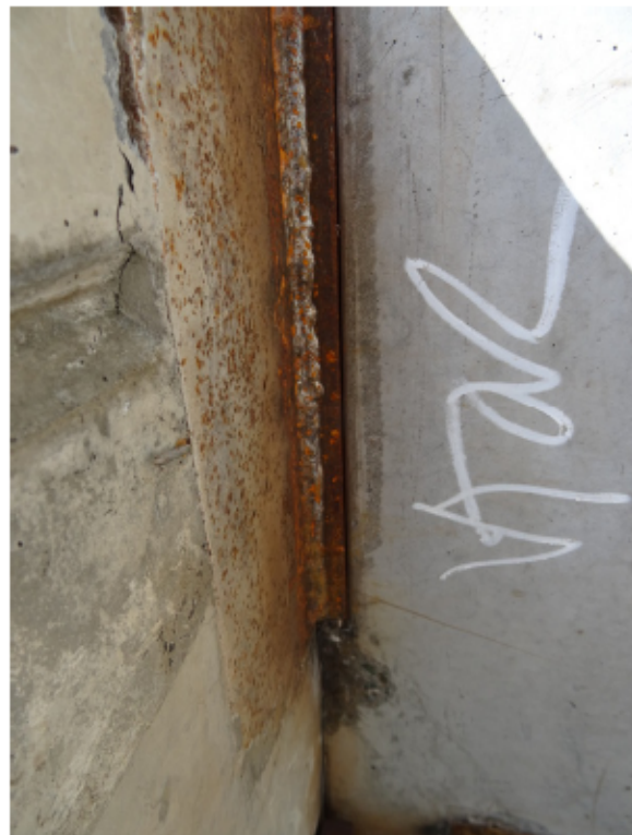
Figure 7: Minor spall at soffit of deck to ballast wall connection (SW)
