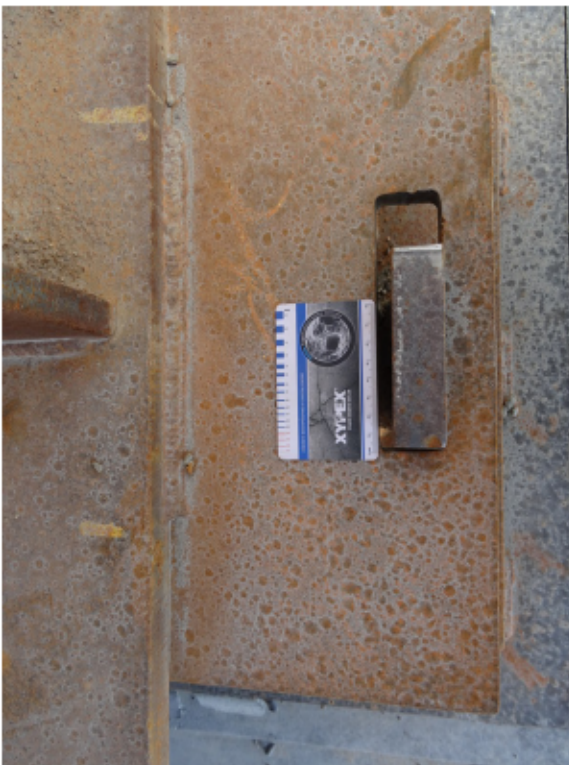
Figure 1: Bearing guide plate nearing end of slot (SW outside of bearing)
