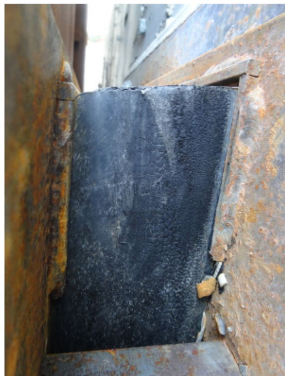
Figure 11: SE bearing front outside face
