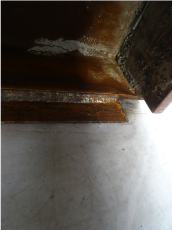
Figure 6: Large weld at ballast wall connection (SW girder, inside face)
