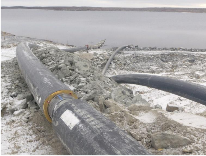
1.1 Whale Tail South diffusers, extended on the shore. Note the heat traced pipe for the winter diffuser.
