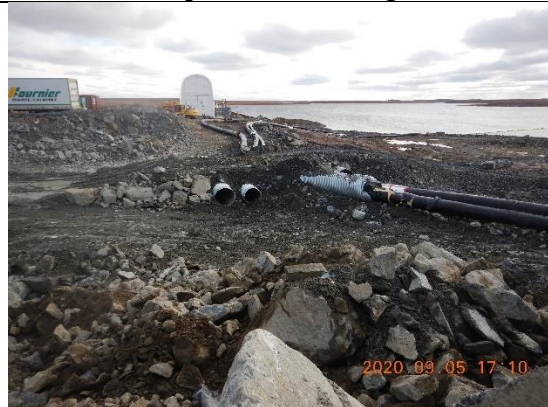
3.4 Culverts installed under WTS Dike access road need to be move uphill to free dike abutment of any material
