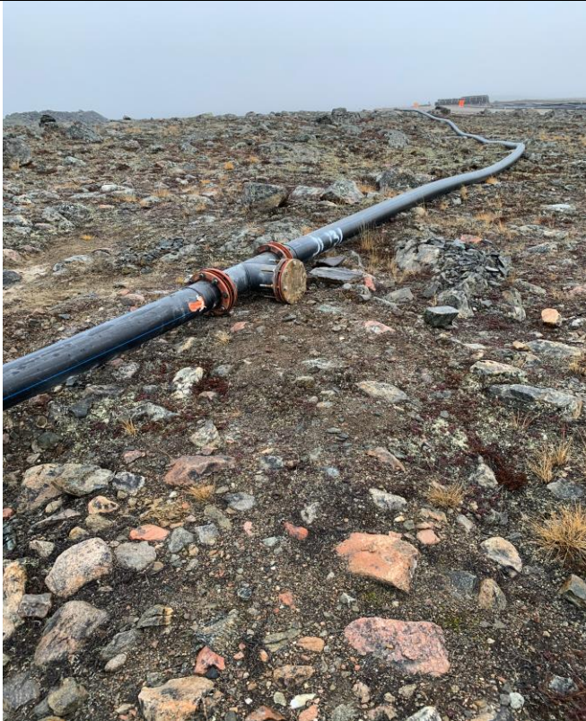
2.1 Missing butterfly valves at the T joint near Nemo Road..
