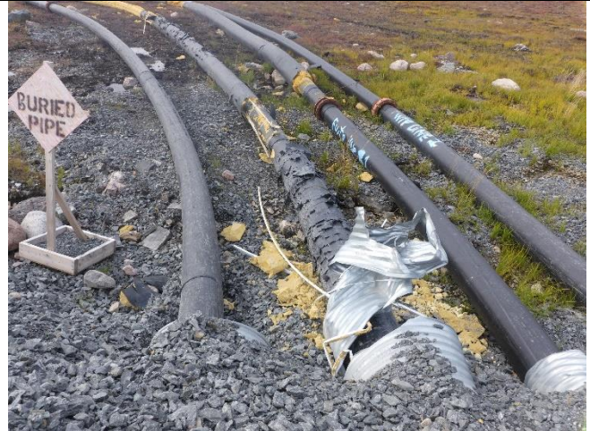
3.2 Torn off insulation layer near the culvert
