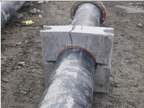
1.1 Tension fracture on a concrete ballast that needs to be changed.
