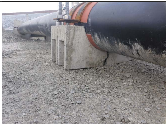
1.1 Fractured ballast that needs to be changed on the winter diffuser
