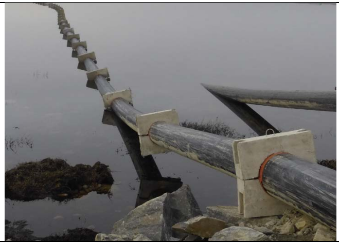
1.3 Ballast on the winter diffuser
