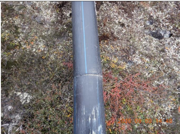
1.2 Pipe misalignment, line 113.
