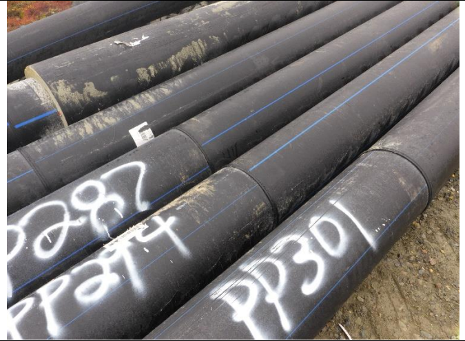
2.1 Adequate fusion observed during a spot check in the pipe stockpile.
