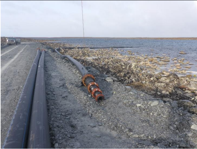
3.1 Diffuser discharging in Mammoth lake and uninsulated pipe on line 140 and 148.
