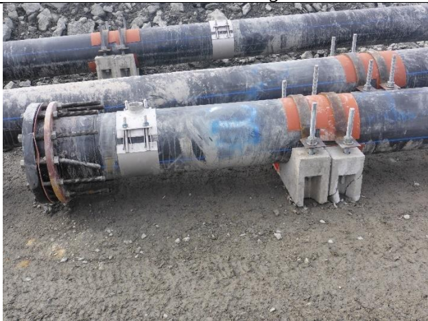
1.3 Bent bolt and slightly broken ballast.
