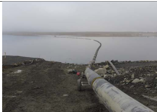
1.1 A section of the winter diffuser in the water
