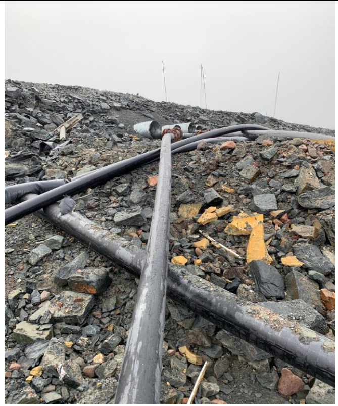
2.2 8" pipe merging into 14" pipe at the culvert between Quarry 1 and WTN
