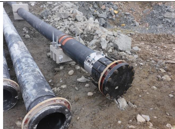
4.4 Adequate pipe ending for the Whale Tail South Lake diffuser
