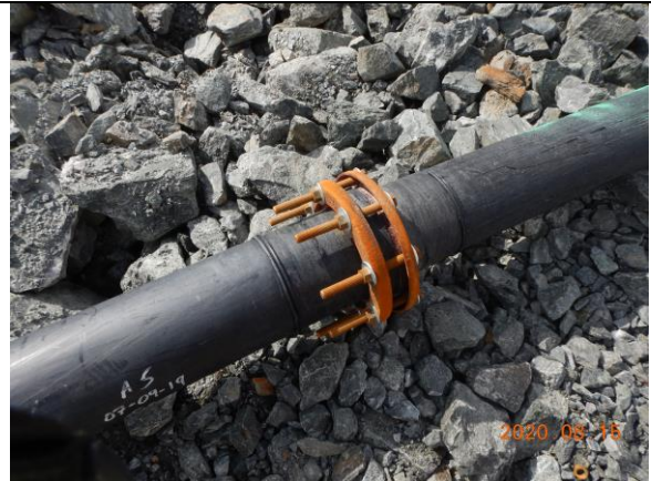
3.2 Flange properly bolted, without gasket Pipe showing damage
