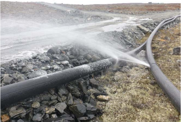
1.2 Pipe cracked between lake A-51 and lake A-53
