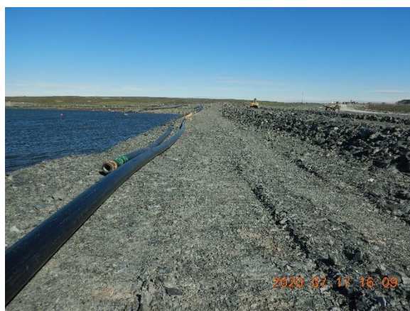
Photo 6. 14" HDPE line 0214 (NE Dike – West Leg)
