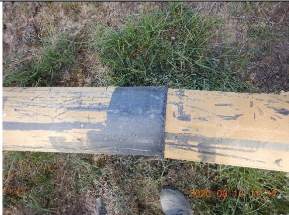
2.1 bad pipe alignment at fusion joint
