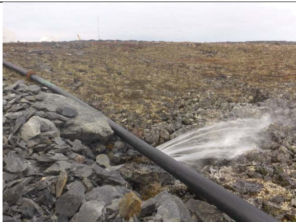
1.1 Pipe cracked between lake A-50 and lake A-53
