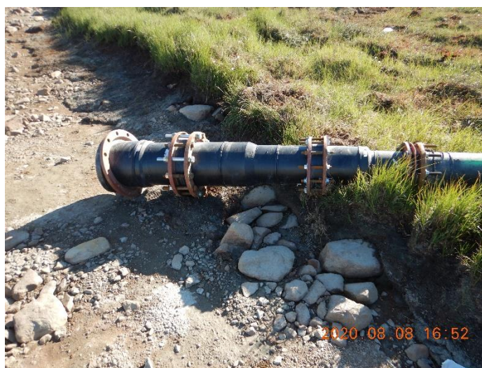
Photo 4. Discharge end Line #0219
