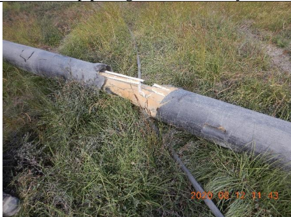
2.3 Pipe laying over electrical cable
