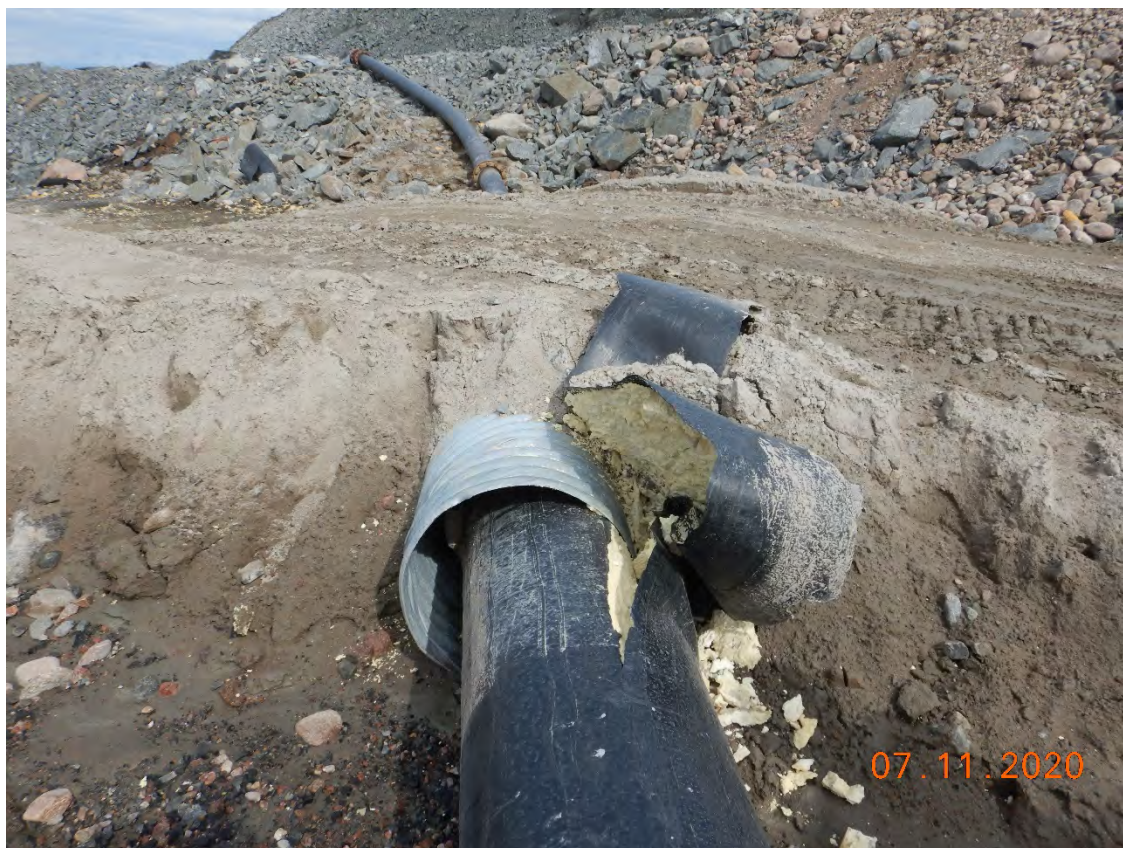
Photo 3. Pipe insulation damaged with the culvert, AP-5
