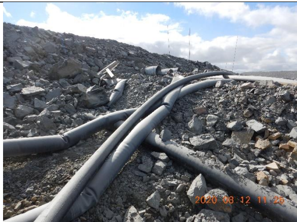
1.6 Mineflex upstream of ring road crossing – squeezed by 8" HDPE pipe
