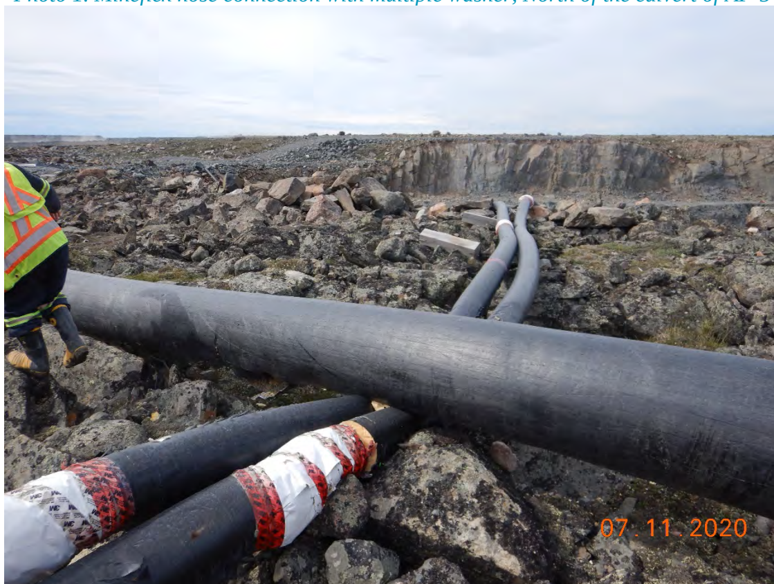
Photo 2. Pipe crossing two smaller pipes, AP-5
