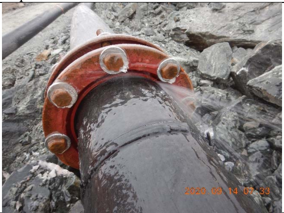
1.4 Flange leaking near lake A-50
