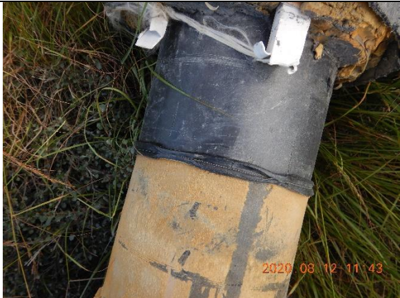
2.2 bad pipe alignment at fusion joint
