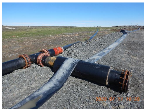
Photo 5. 12" MineFlex Line 0214 (NE Dike – East Leg)
