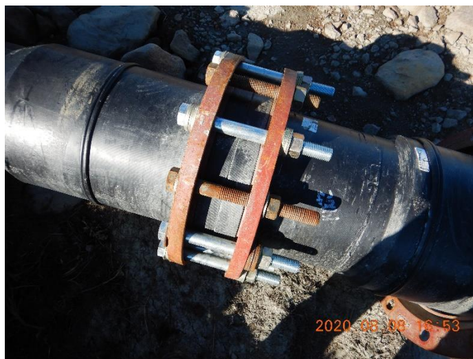
Photo 3. Flange connection Line #0219
