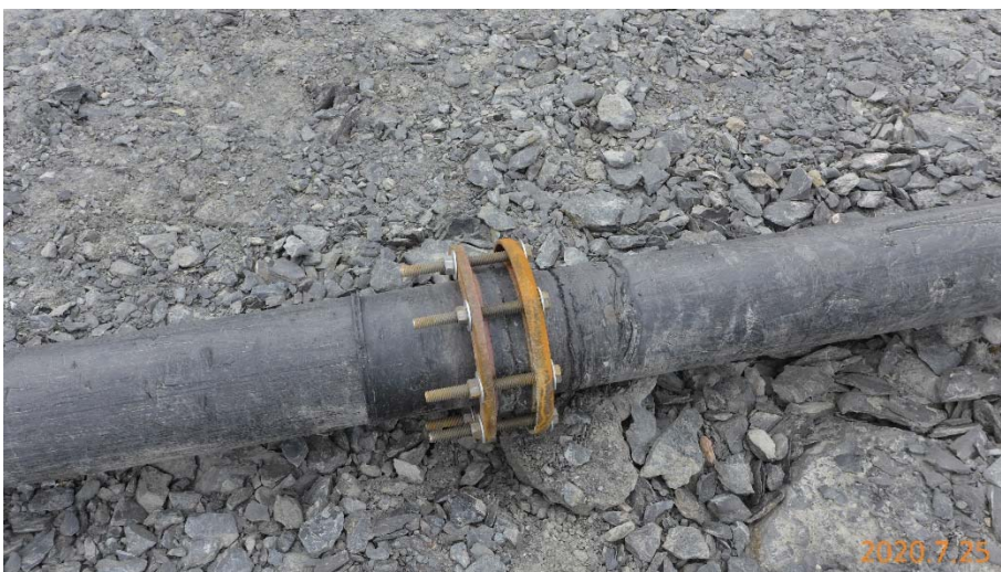
Photo 3. Flange connection Line #0217
