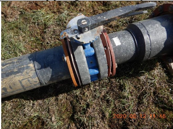
2.4 Insufficient bolting at valve connections
