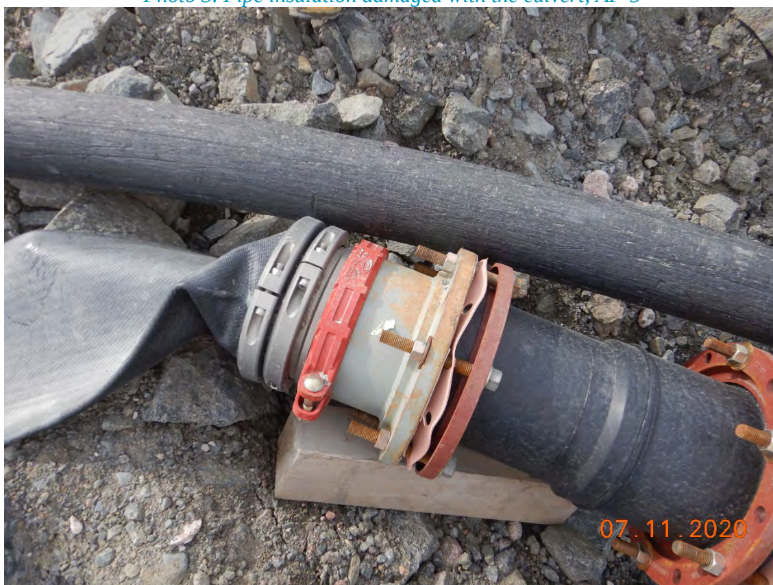
Photo 4. Missing bolts at a Mineflex connection, beside the pit ramp culvert
