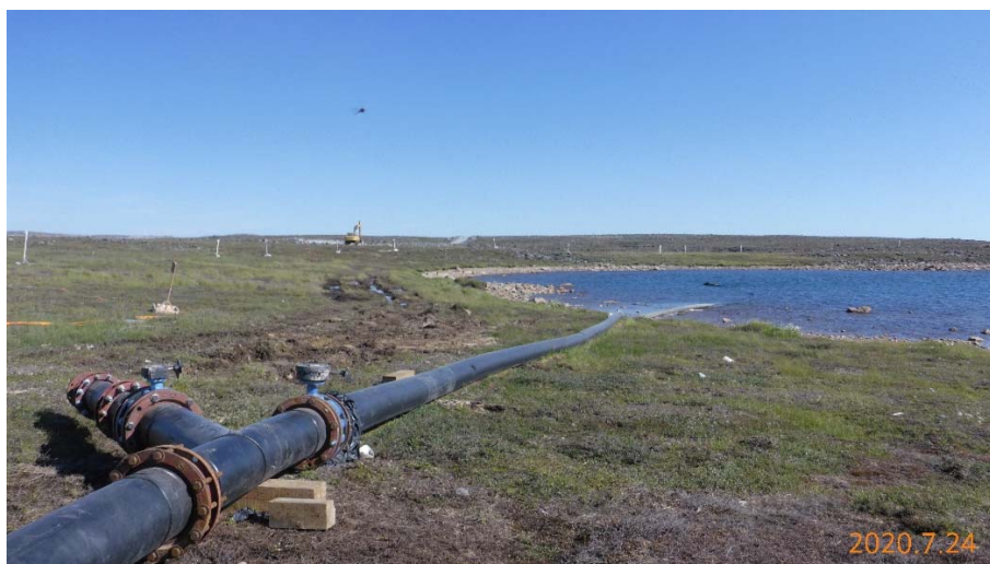
Photo 1. Y on the suction of the Line #0211
