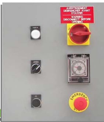
Figure 2 -- Brome Composter Control Panel
