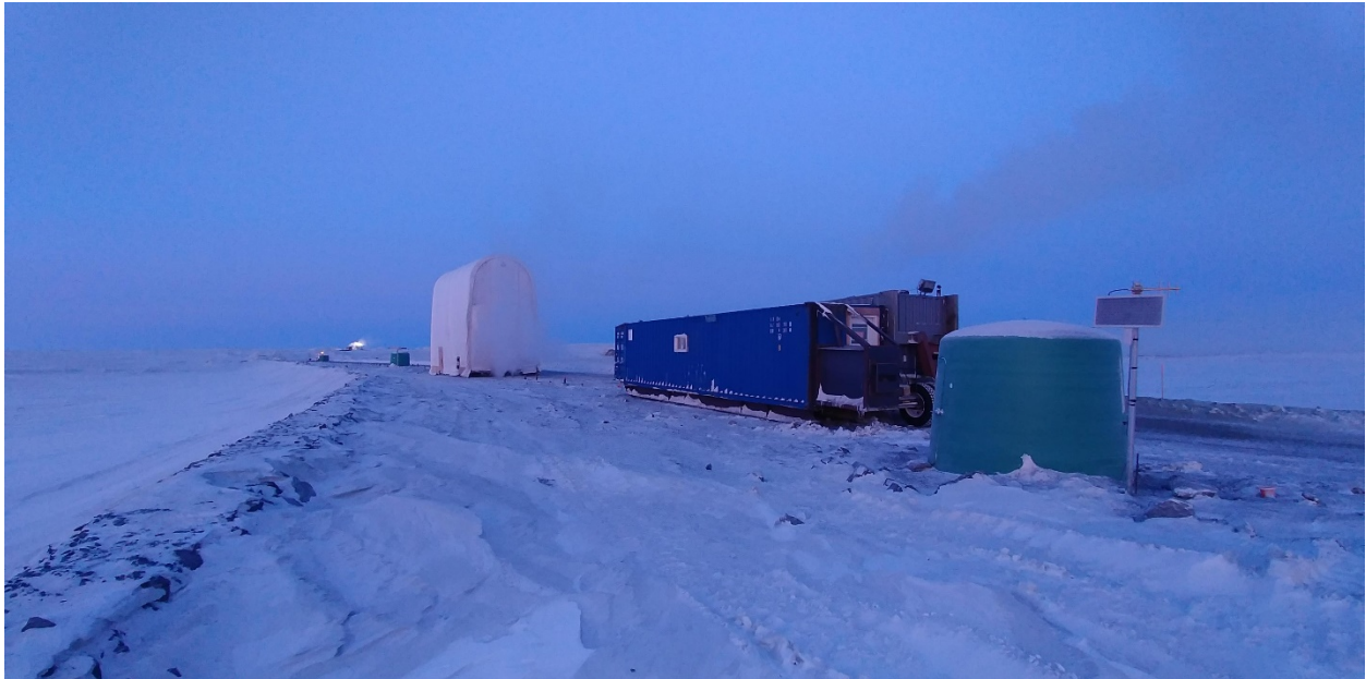
Photo 1: View of the WTD with injection unit and drilling rig dome
