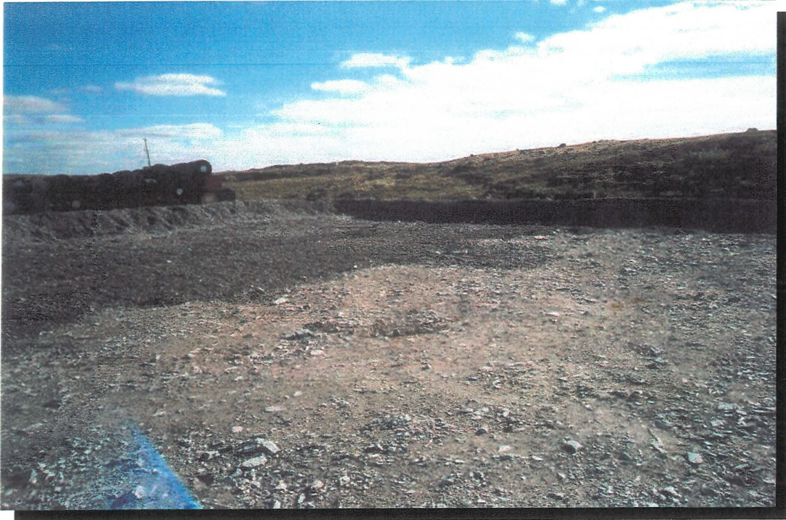
Photo 12 Photograph of crush material used as bedding for landfarm area. Looking south.
