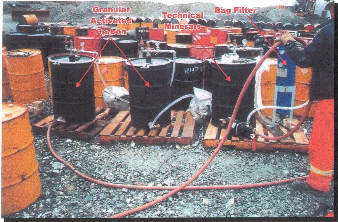
Photo 15 Photograph of water treatment system.
