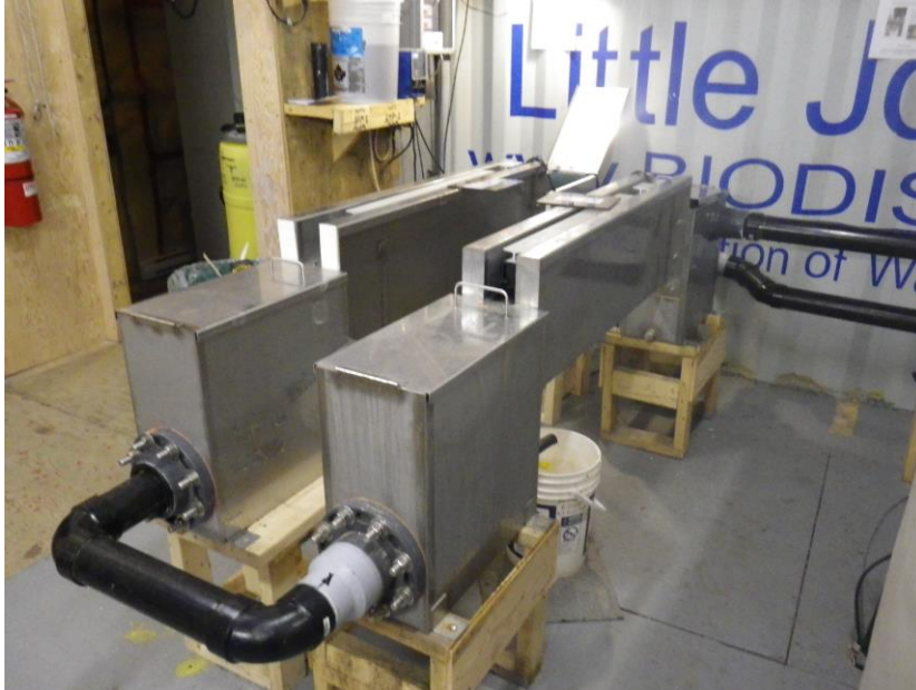
Figure 2: 2 UV water disinfection systems
