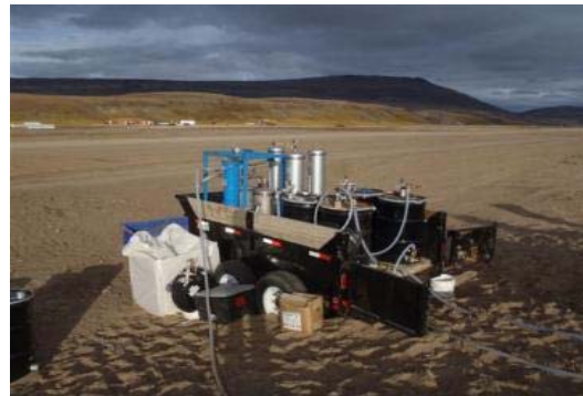
Photo 5: Mobile oily water treatment system at the Mary River bulk fuel storage facility.
