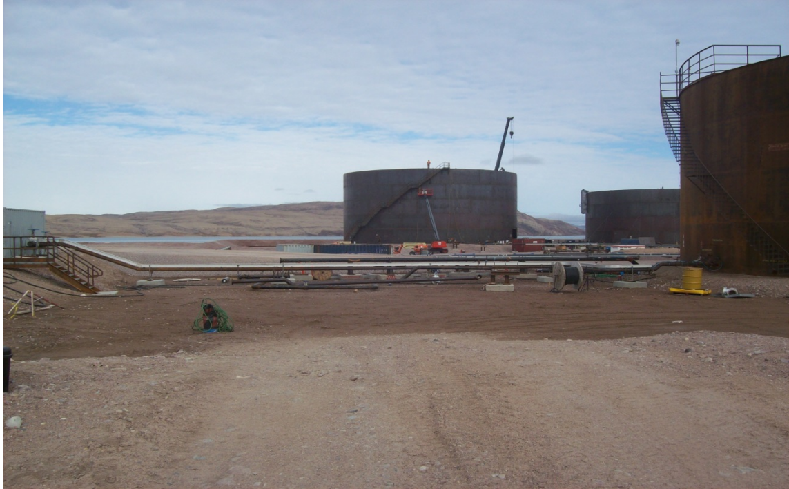
Containment area (1 only 12 M litre tank in foreground and 2 only 5M litre tanks in background)
