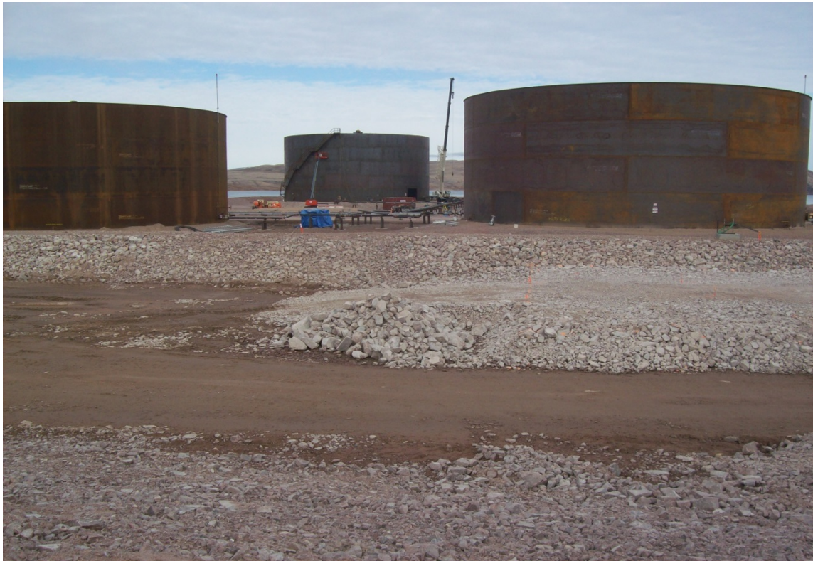
Central part of Fuel Tank Farm with pads for 0.75 M litre jet fuel tanks in foreground and 12M litre fuel tanks in background
