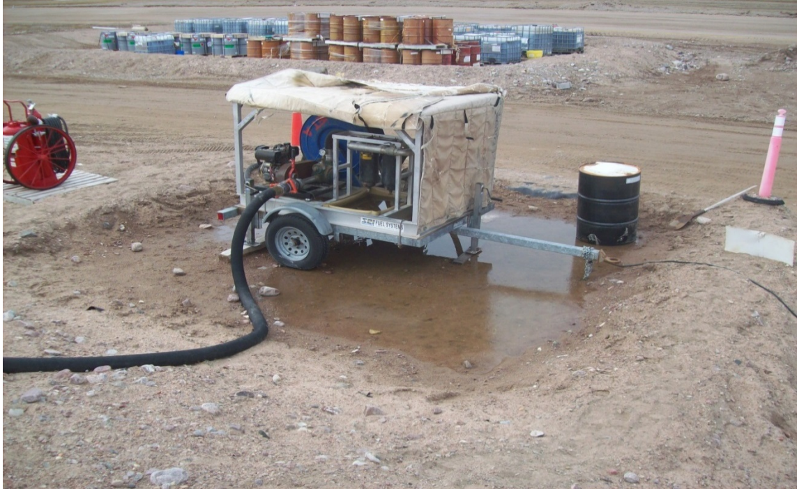
Jet "A" Pump Containment
