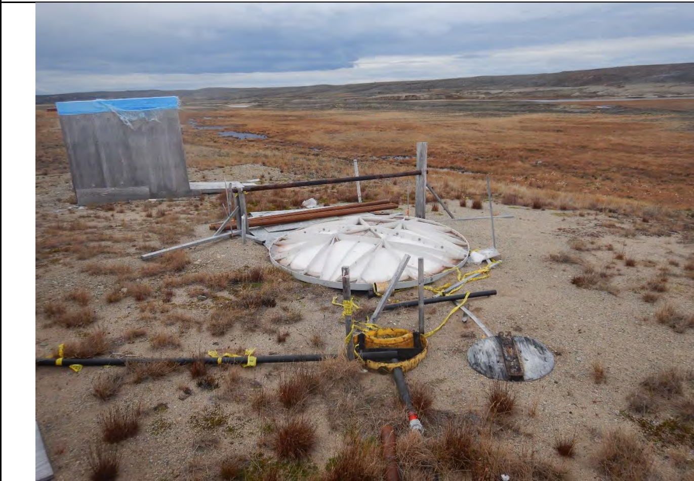
Description: sump without berms to prevent flooding.
