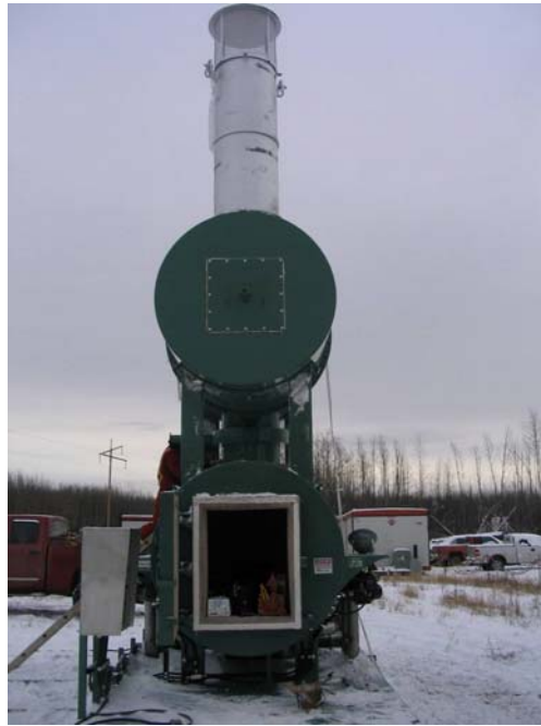
Figure 2.2 Typical Controlled Air Dual Chamber Incinerator
