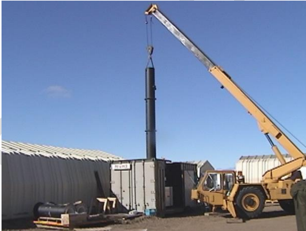
This is a Sample Photo only of Erection of the Stack Sections
