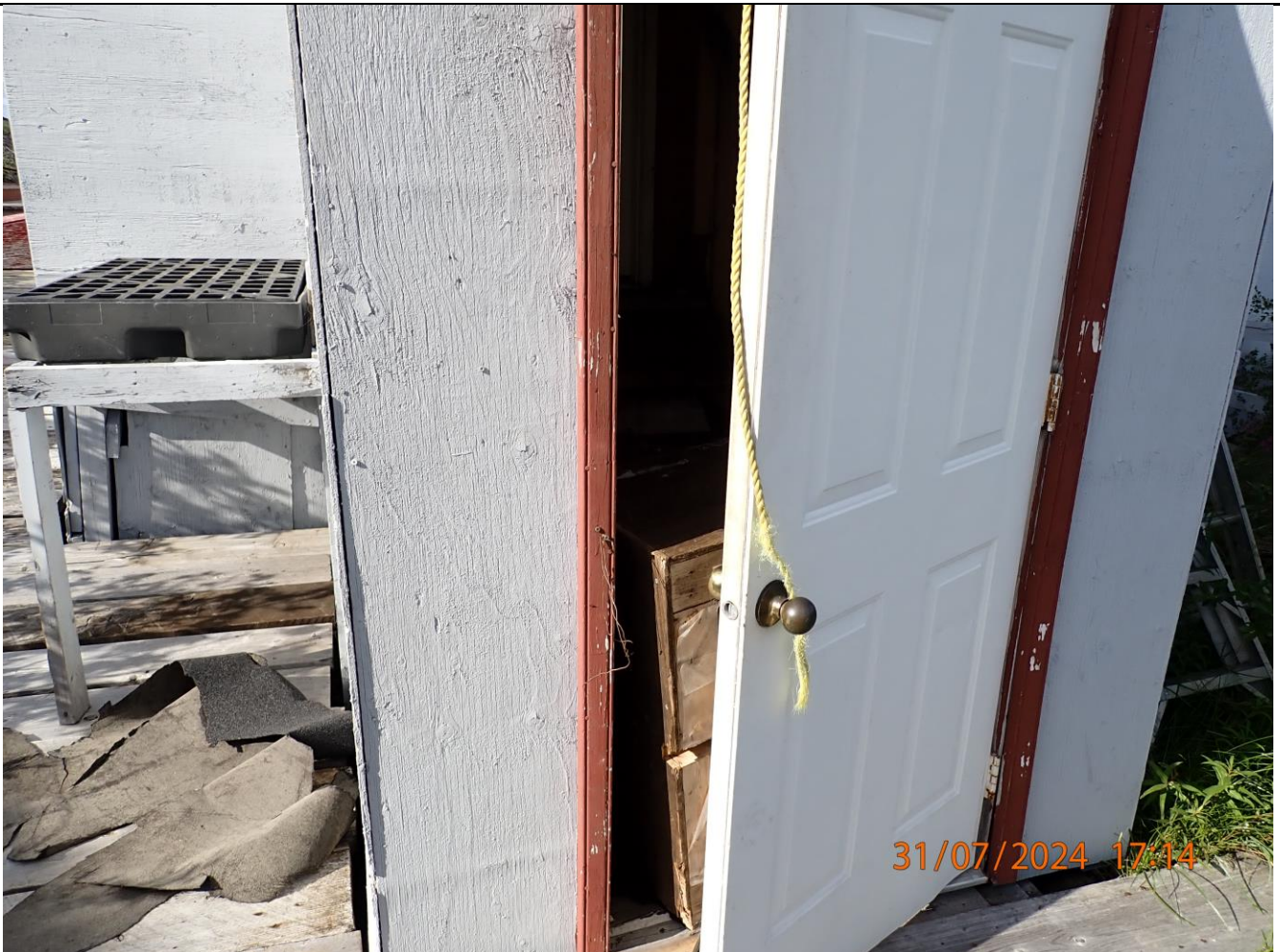
Roofing material outside main building, image shows box in door way. Bear sign is apparent in the building.
