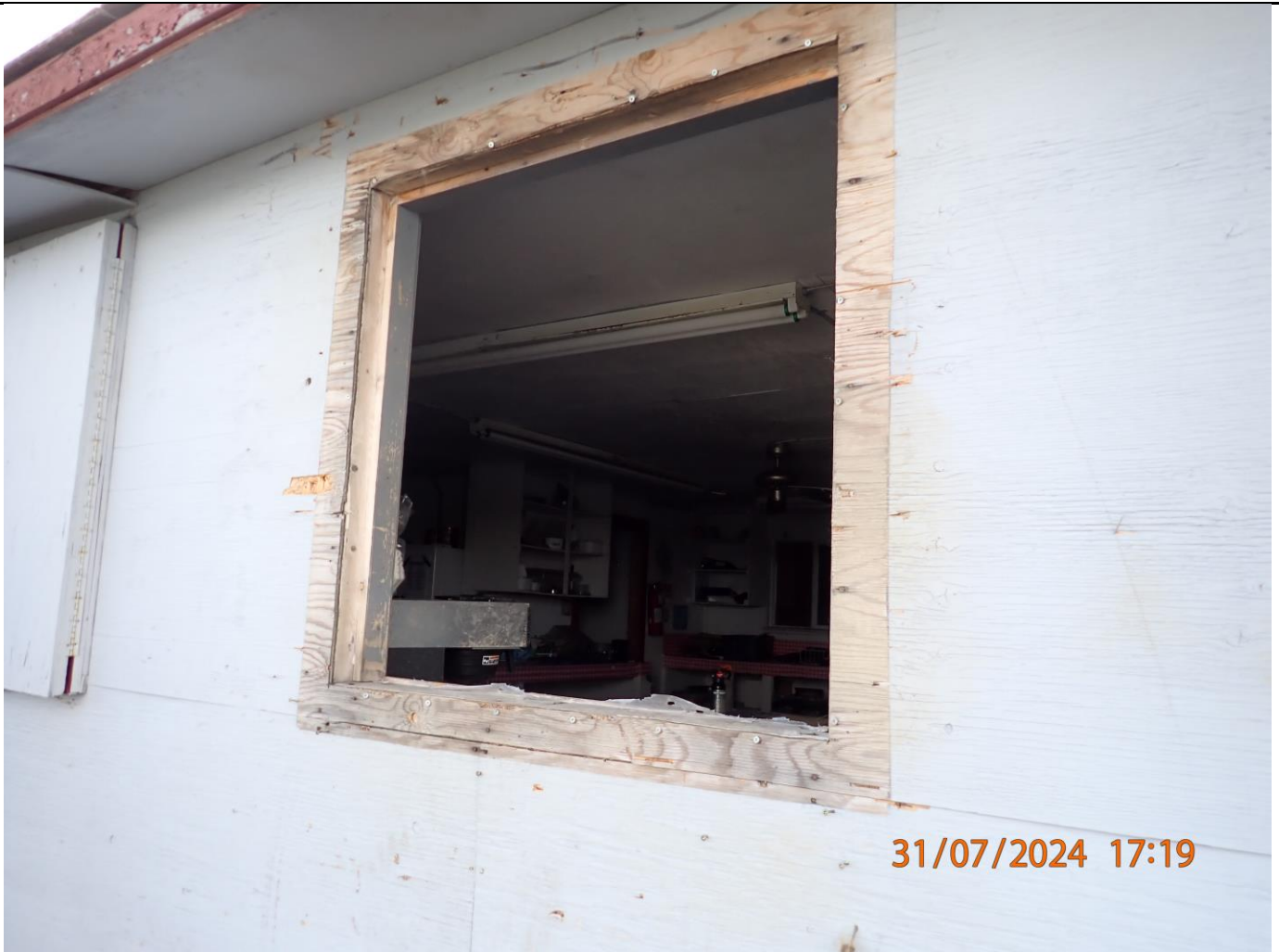
Main building kitchen window open, the plywood was observed on the ground.
