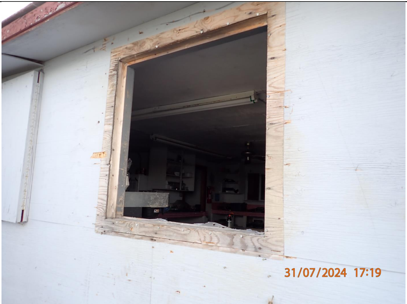
Main building kitchen window open, the plywood was observed on the ground.
