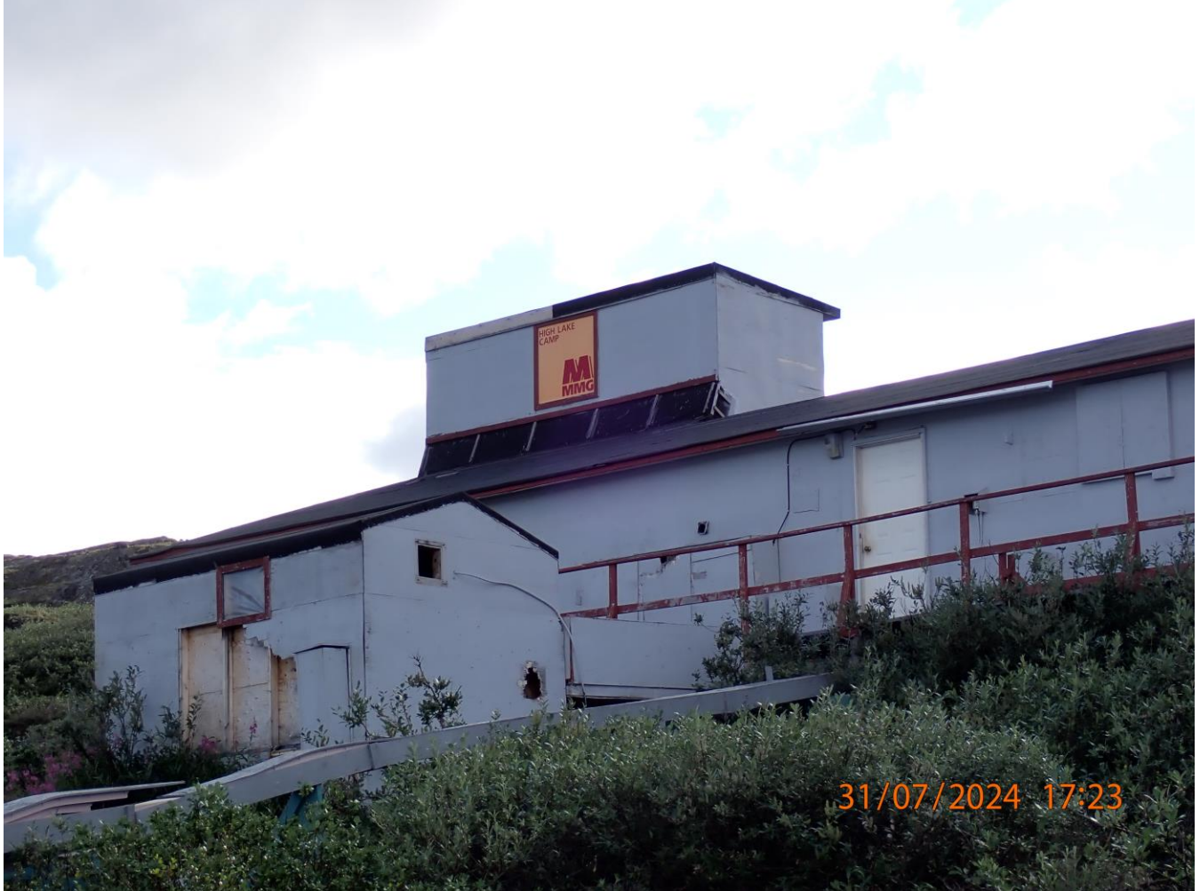
Another view of the shack beside the main building, Plywood from the wall is missing, an open window and a hole in the back wall is shown.
