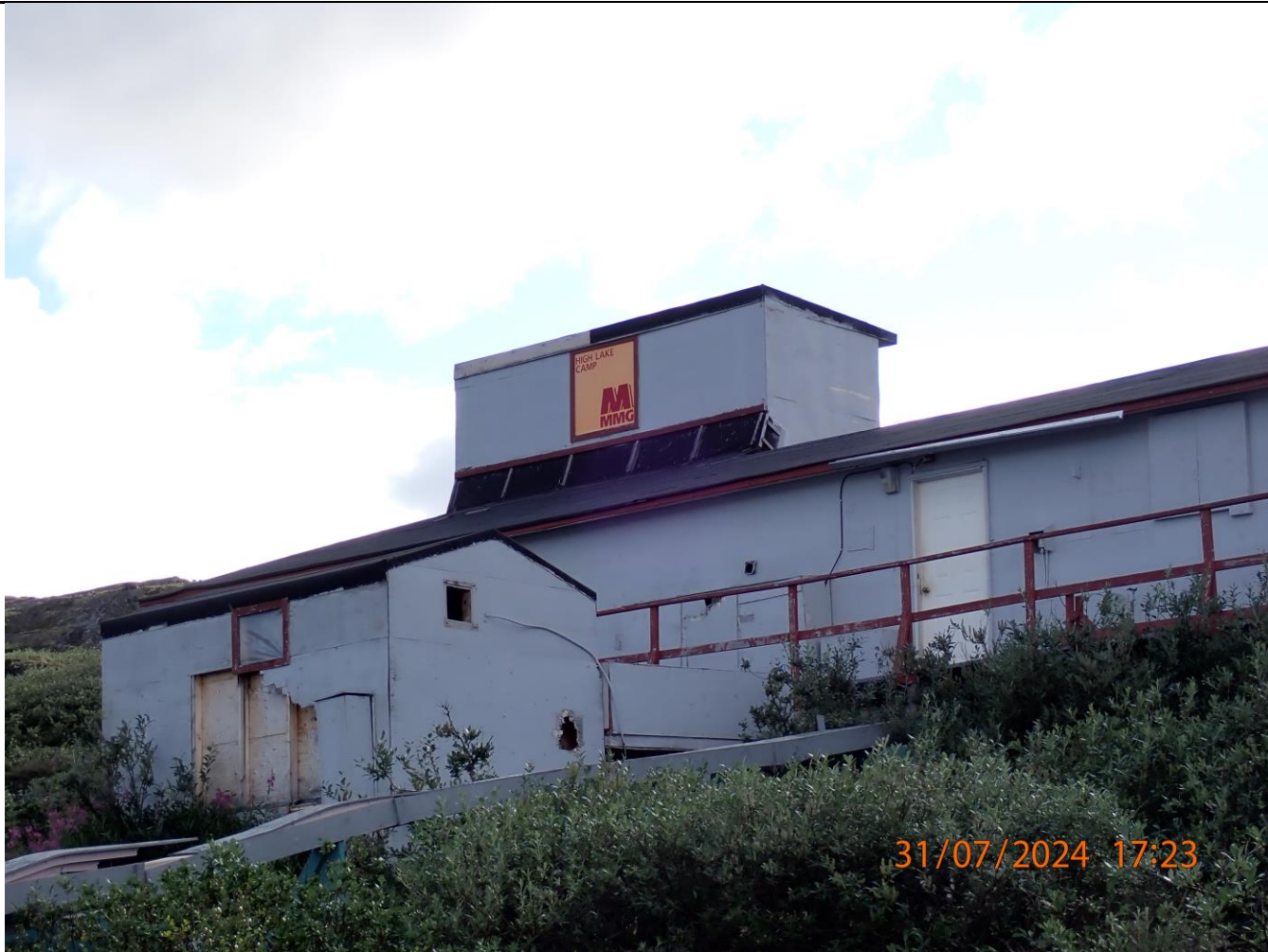
Another view of the shack beside the main building, Plywood from the wall is missing, an open window and a hole in the back wall is shown.
