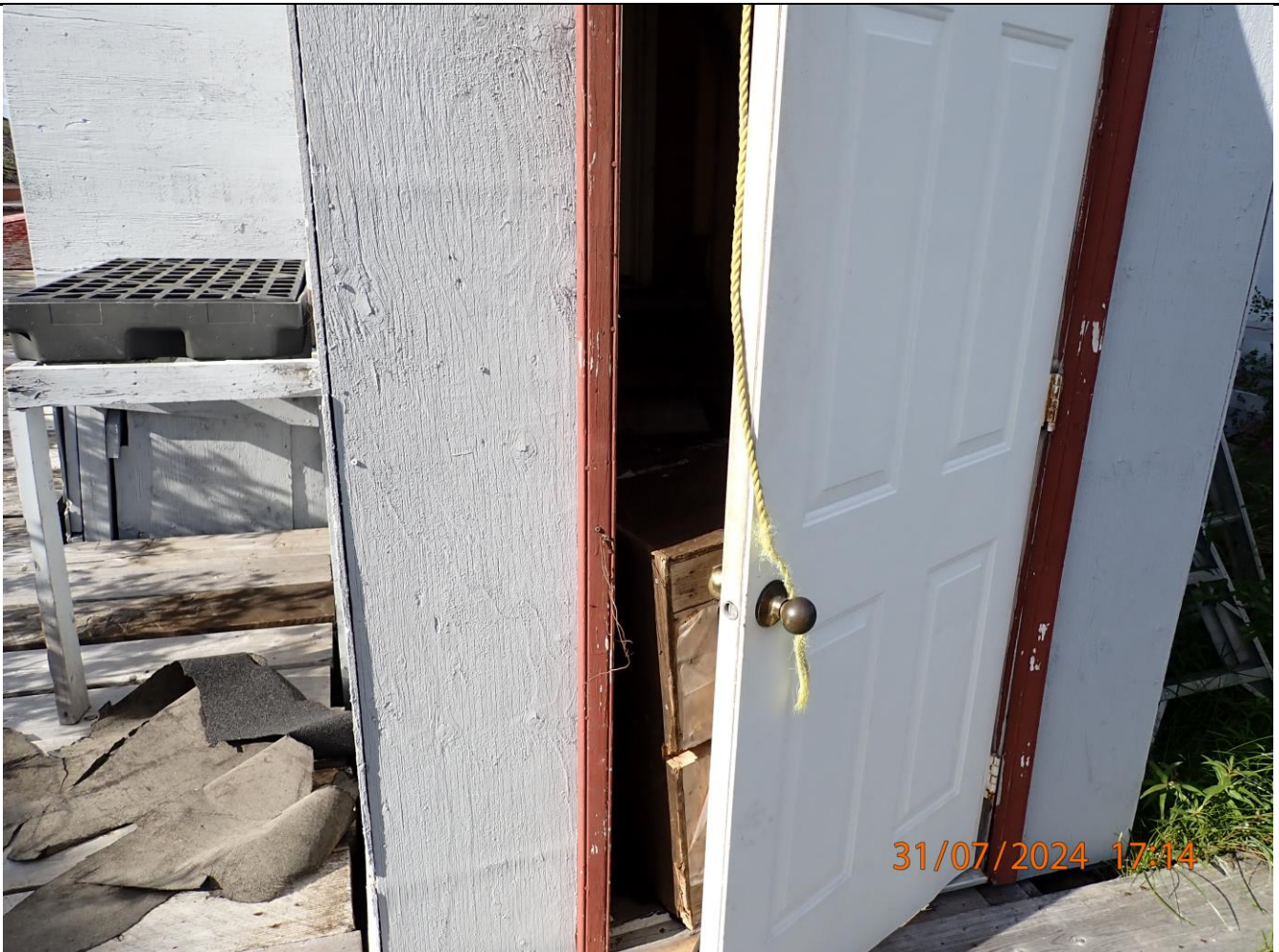
Roofing material outside main building, image shows box in door way. Bear sign is apparent in the building.
