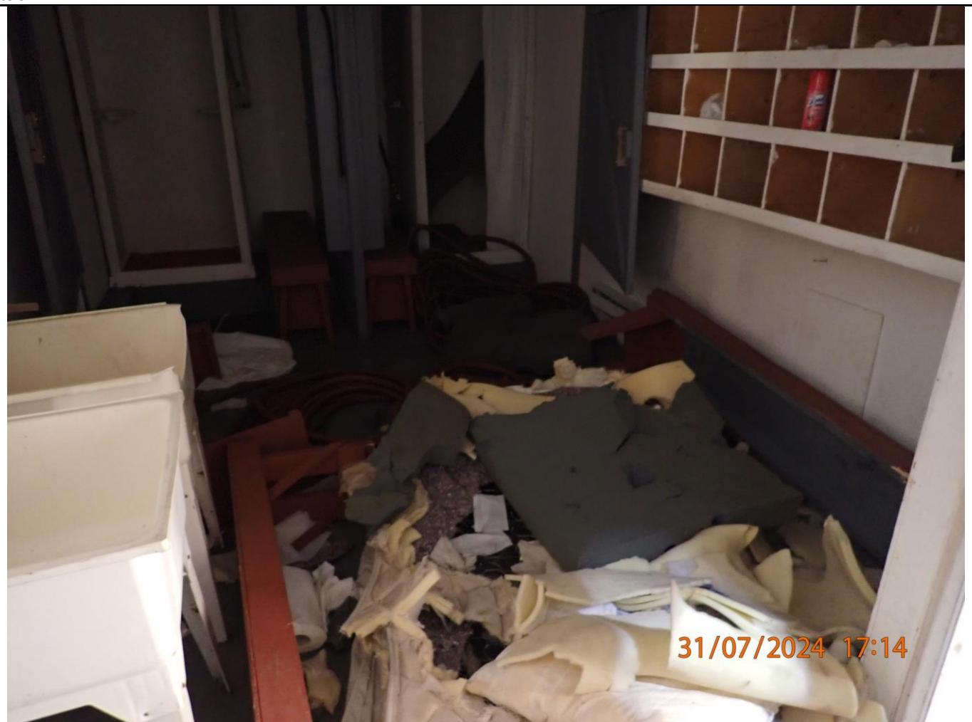
Inside the main building entrance, mess caused by a bear
