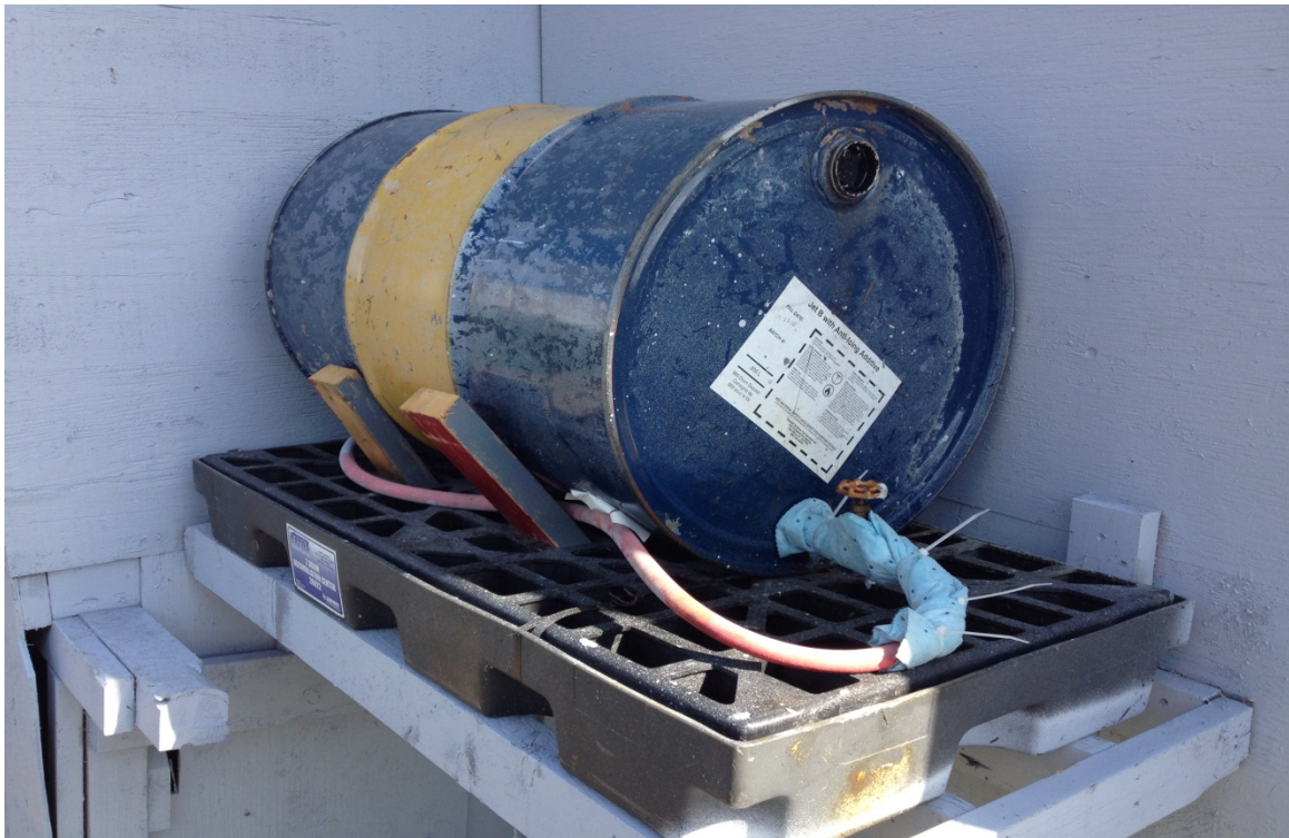
Secondary Containment at Stove Fuel Supply – Kitchen High Lake
