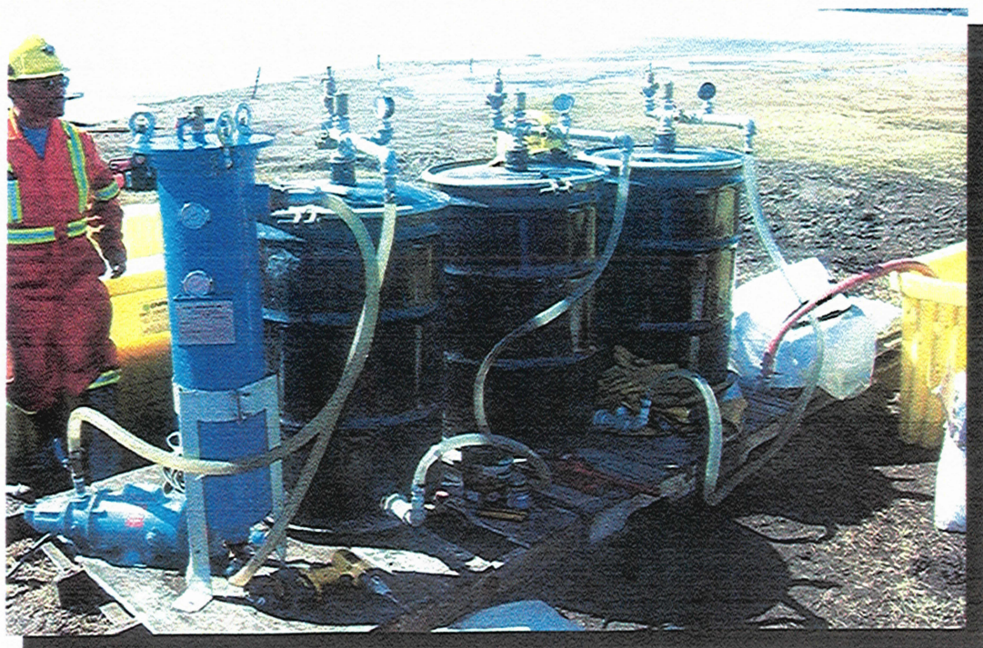
Photo 18 Water treatment system.
