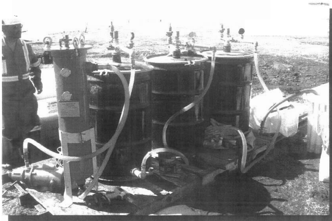
Photo 18 Water treatment system.
