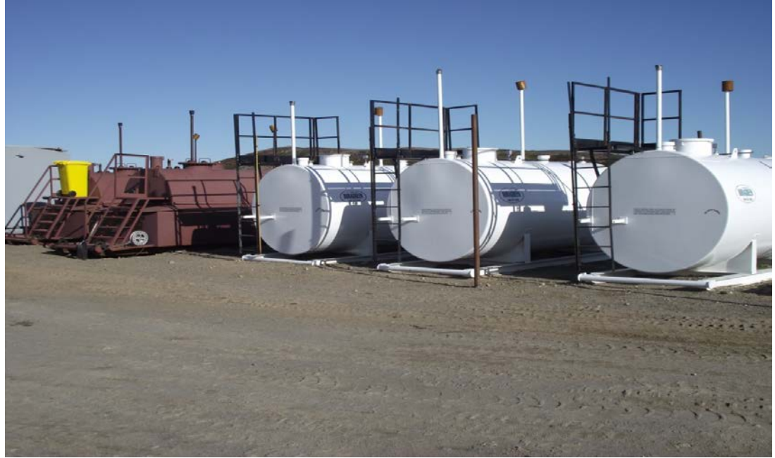
Fuel farm 11,000L double walled storage tanks with spill kit – August 2011
