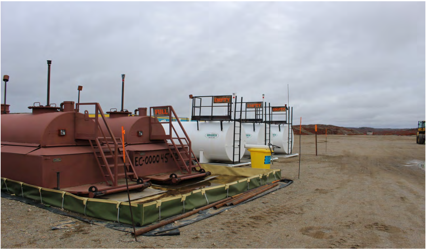
All of the remaining bulk tanks have now been drained.
