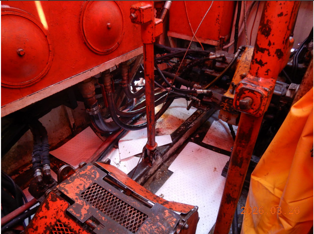
Description: Spill pads under hydraulic components of operating drill.
