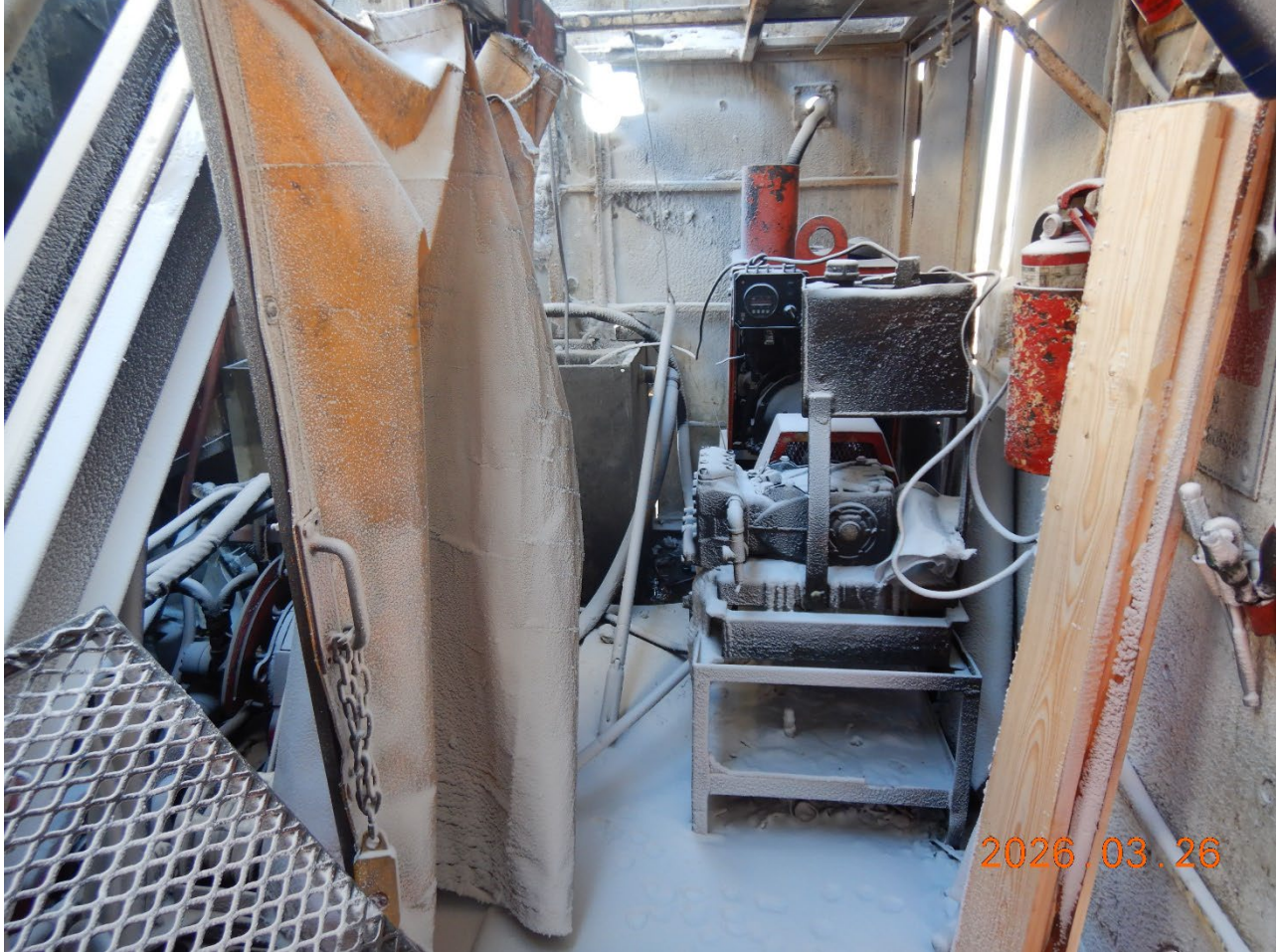
Description: Spill pads under components of laid up drill.
