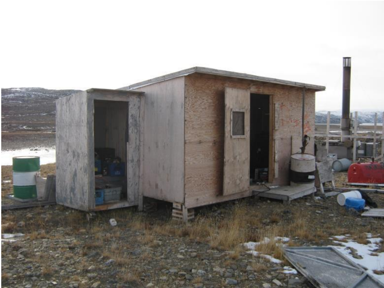
Figure 17 – Shed and attachment with open/ missing doors
