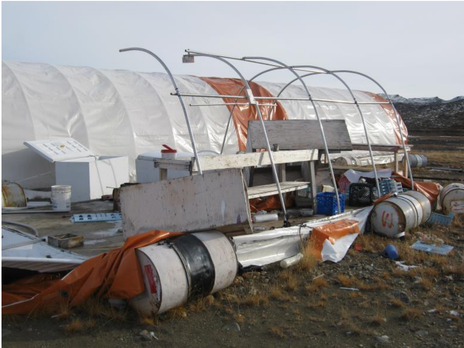
Figure 4 –Damaged hut and exposed interior
