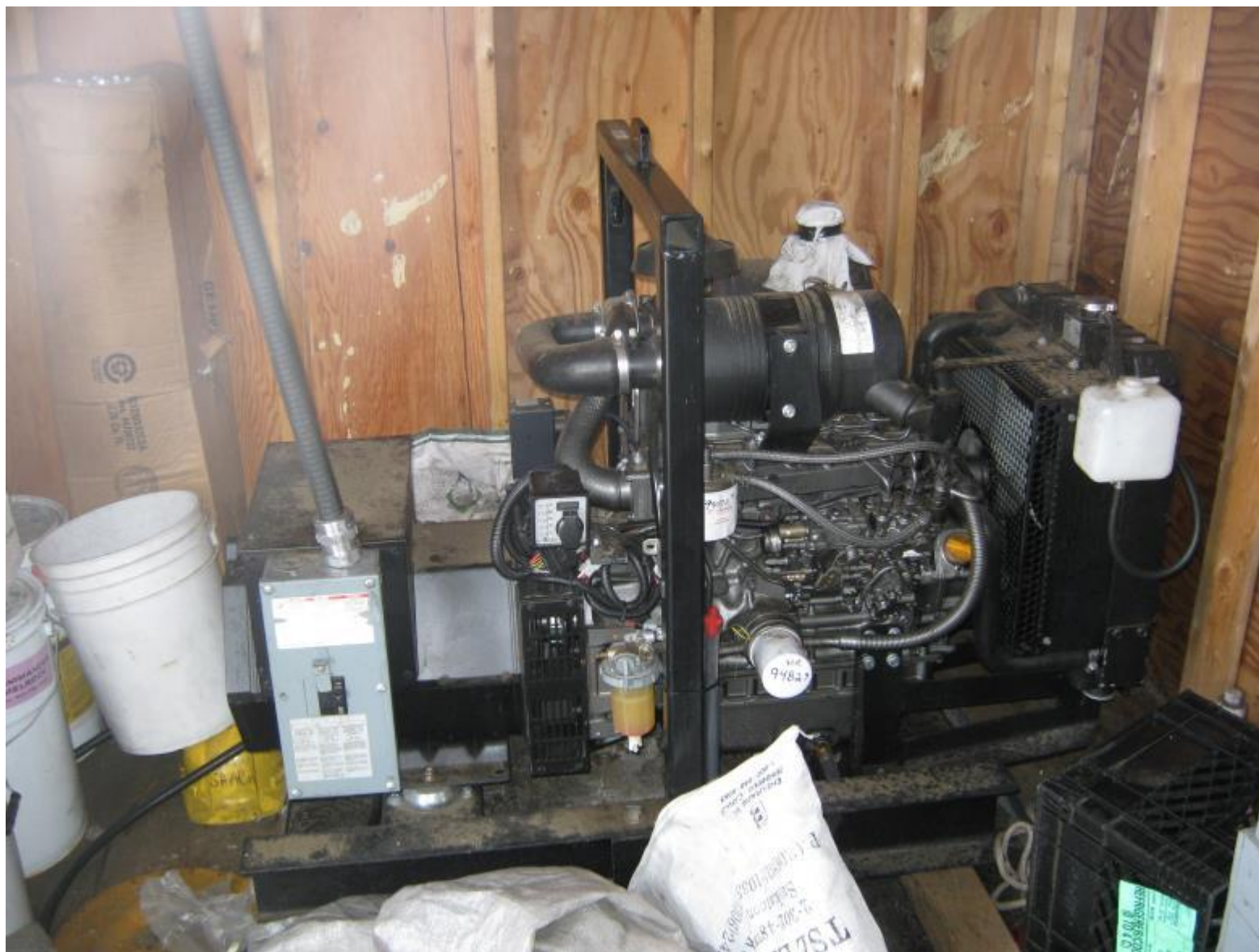
Figure 18 – Generator 1 in shed
