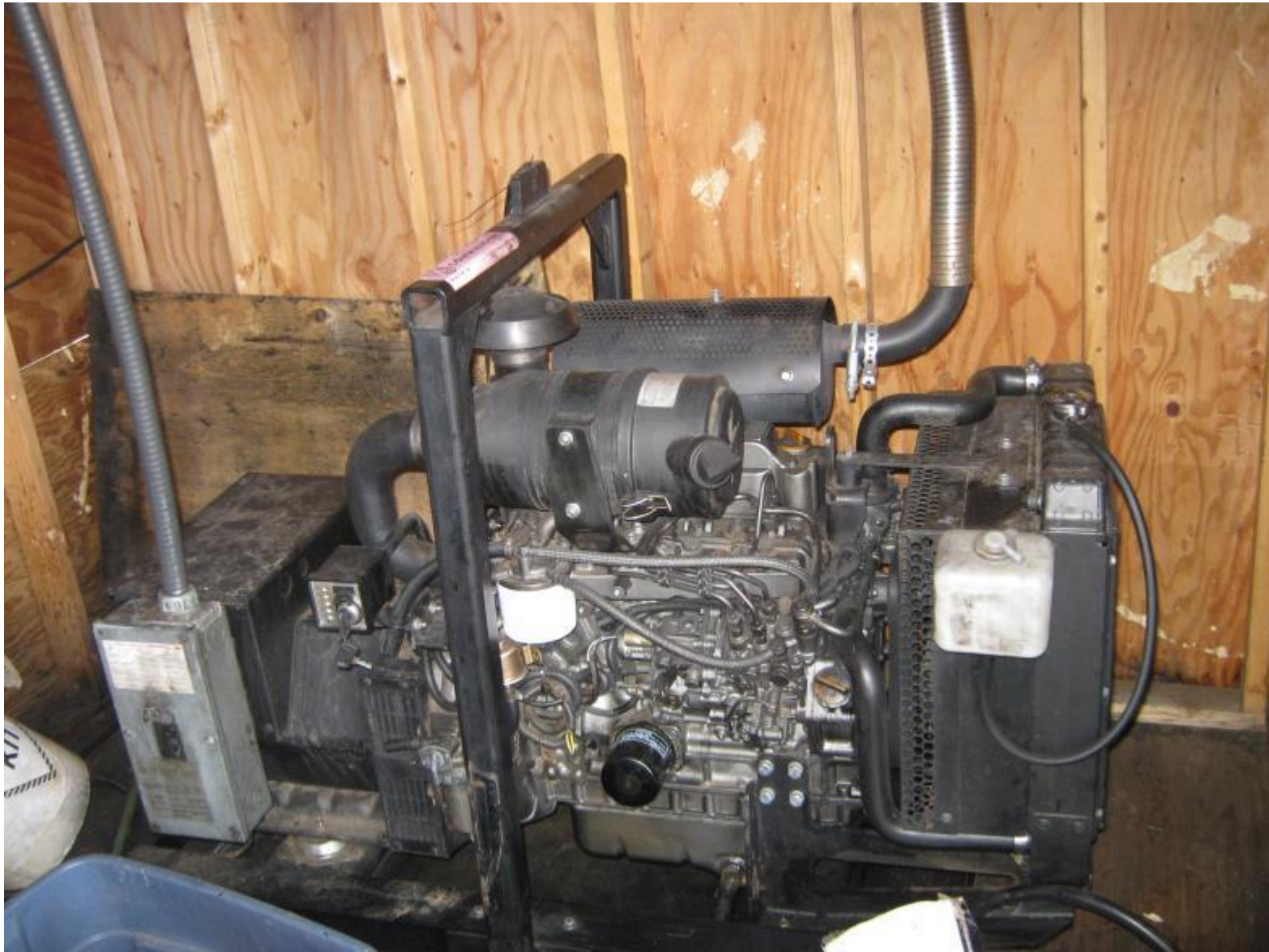
Figure 19 – Generator 2 in shed
