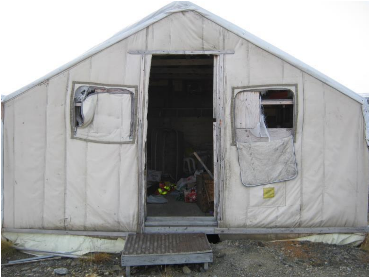
Figure 3 – Partially damaged hut
