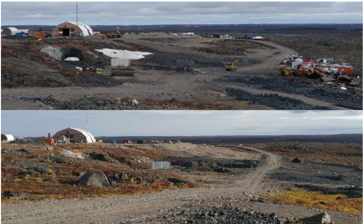
Photo 4. Ulu landfill area, before and after.
