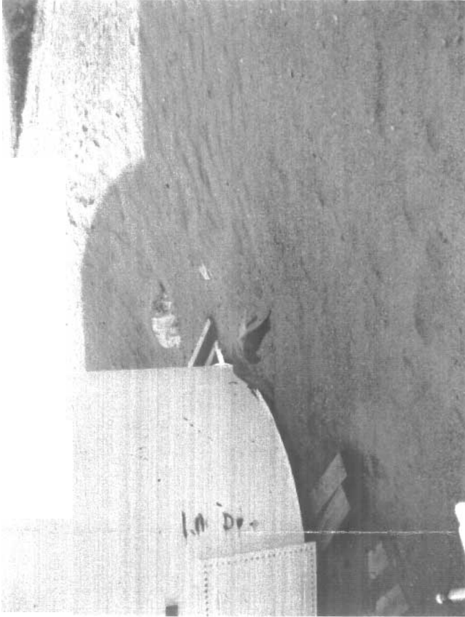
Photo shows some exposed liner right at the bottom of the stand up tanks.
