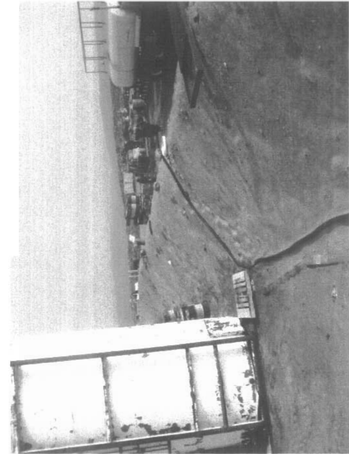
Photo shows a view of the inside of the main tank farm. The liner is exposed where the sand has been eroded off the inside face. The liner should be covered up.
