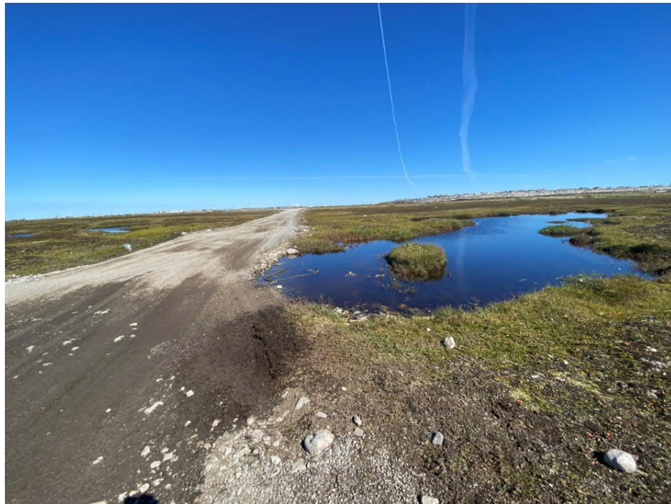
Figure 4: Gravel roadway and pooled water northwest of the WTA
