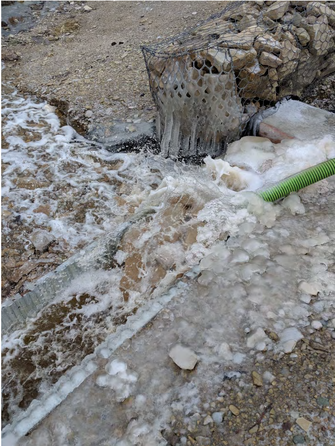
Photograph #3: Pump outlet.
