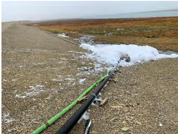
Decanting pump in operation Downstream - Outlet
