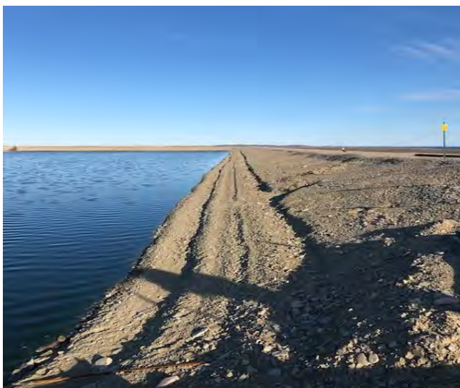
Collapsing interior berm soil within cell “A”
