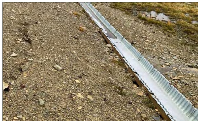
(b) Photo of Trough at Cell B
