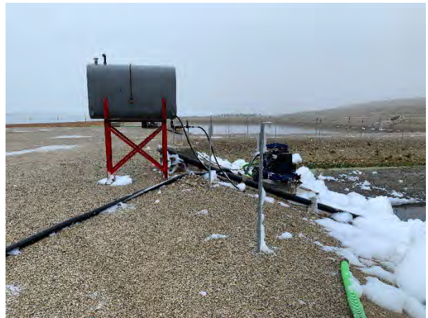
Decanting pump in operation Upstream - Inlet
