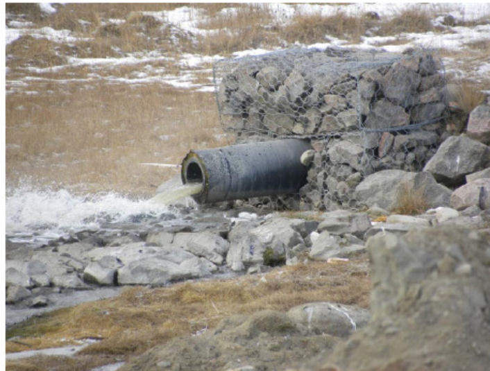
Photograph 6 Discharge from Sewage Treatment Plant
