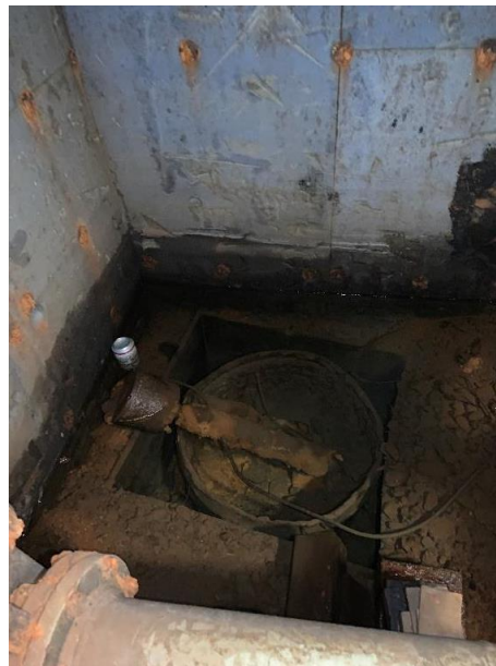
Figure 11: Sump pump and pit in the southwest corner of the Access Vault (VR Associates Inc., 2023)
