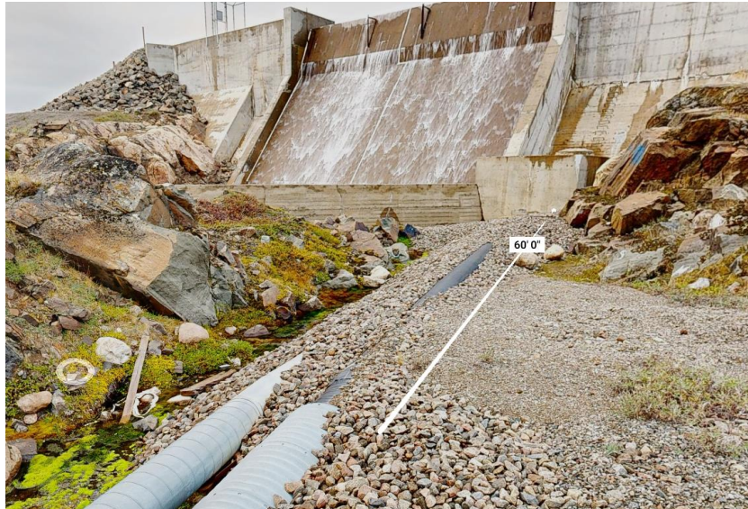
Figure 8: Intake Piping from Access Vault
