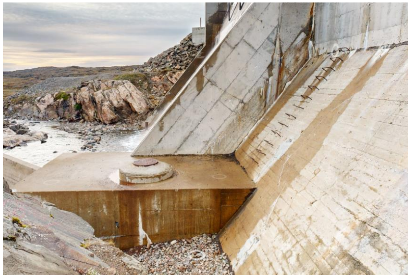
Figure 5: Lake Geraldine Access Vault
