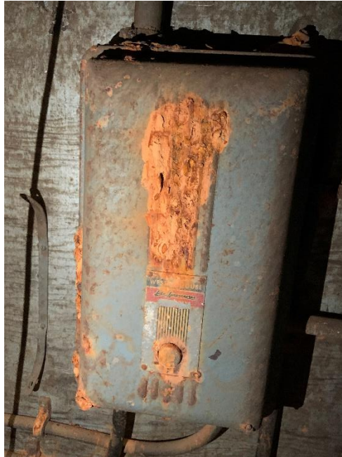
Photo 2.1.3: motor starter, assumed to be wired to sump pump
