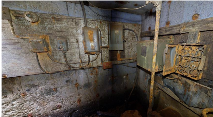
Figure 12: Electrical System Components Along South and East Walls
