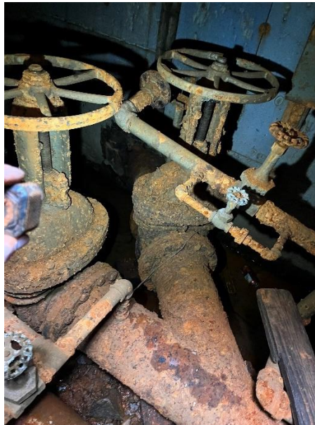
Photo 2.1.2: Example of heavily corroded piping and valves
