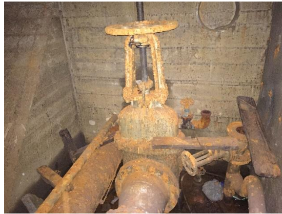
Photo 2.1.1: Example of heavily corroded piping and valves.
