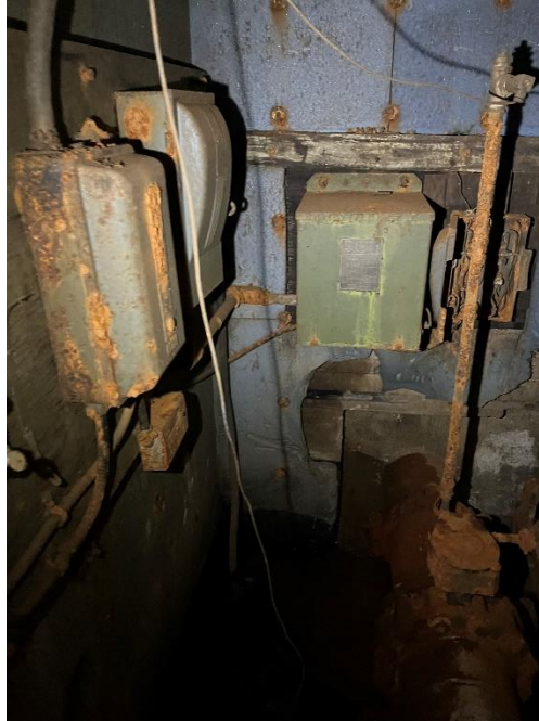
Photo 2.1.2: overall view of existing electrical services
