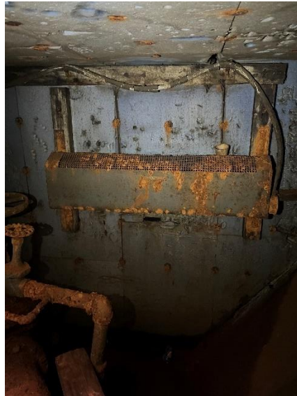
Photo 2.2.1: existing electrical radiant heater
