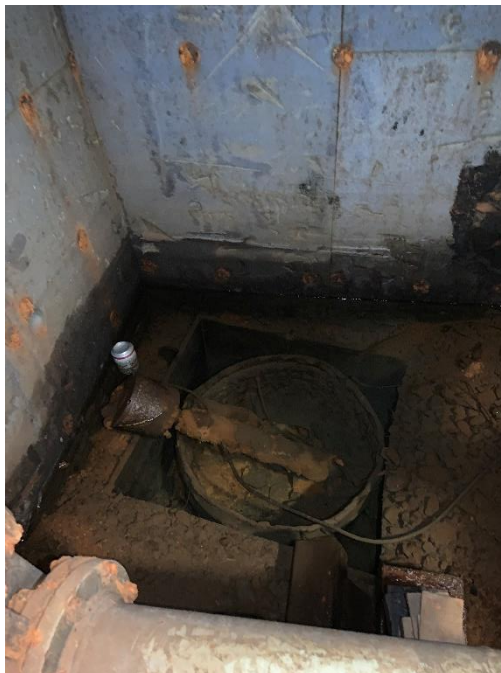
Photo 2.1.5: Sump pump and pit
