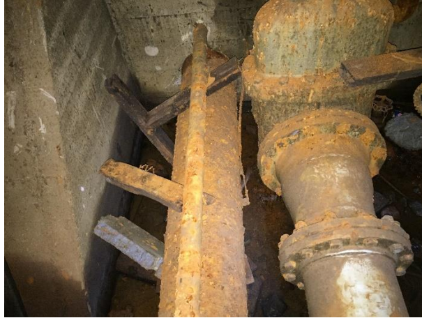
Photo 2.1.4: example of scrap metal propping up piping
