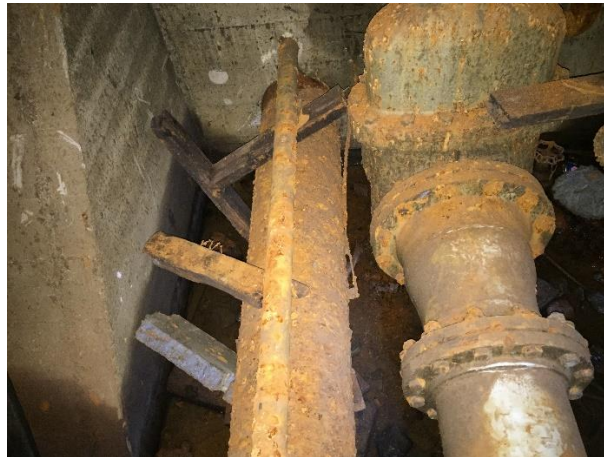
Photo 2.1.4: example of scrap metal propping up piping
