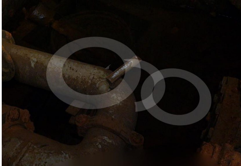
Figure 10: Corroded Sensor on Heated Water Line
