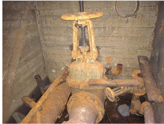
Photo 2.1.1: Example of heavily corroded piping and valves.
