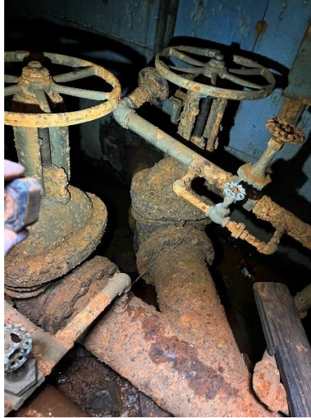
Photo 2.1.2: Example of heavily corroded piping and valves
