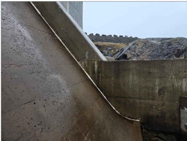
Figure 38 Left Training Wall Sealant Intact
