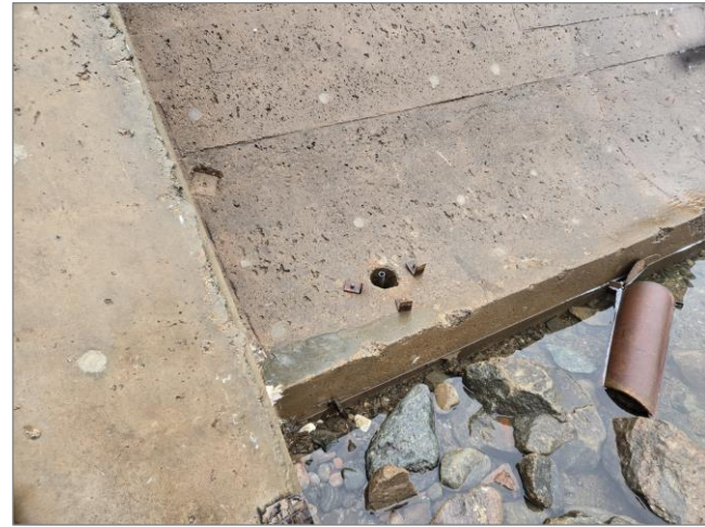
Figure 24 BH112, Piezometer Exposed
