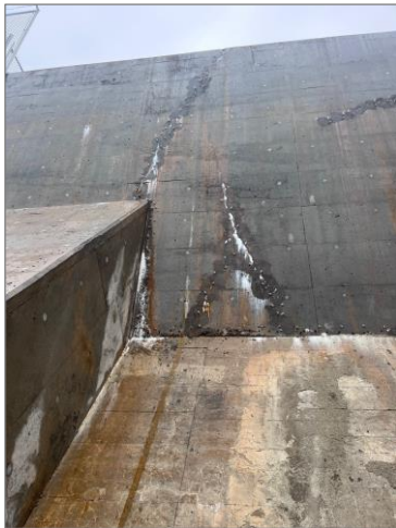
Figure 46 Crack Repair – Injectors Not Cut Flush
