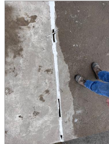
Figure 48 Expansion Joint Sealer - Removed by Rodents
