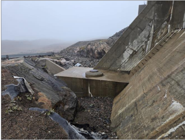
Figure 33 Intake Valve Chamber
