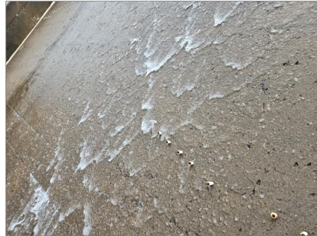
Figure 39 Protruding Caps to be Removed
