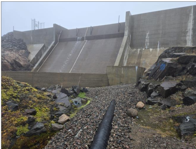
Figure 34 Exposed Waterline to Treatment Plant
