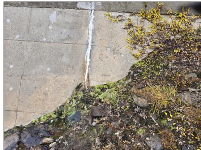
Figure 44 South Concrete Dam Seeping at Foundation
