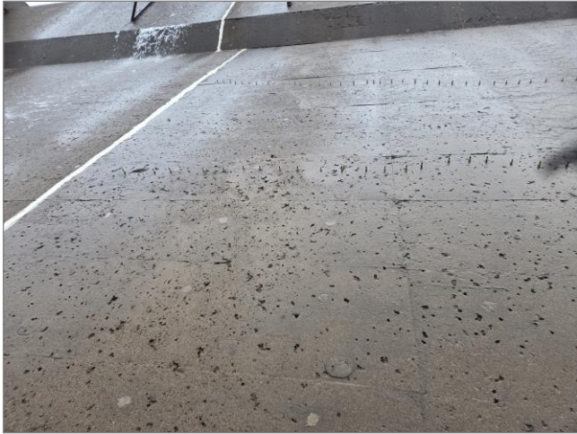
Figure 37 Porosity in Spillway Conveyance Surface
