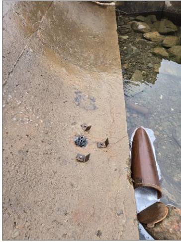
Figure 25 Spillway Apron, BH113 Piezometer Exposed
