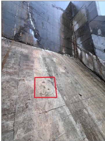
Figure 19 Spillway Spall Location
