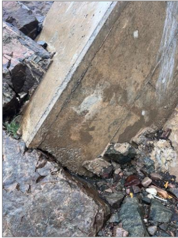
Figure 45 Minor Seepage at Concrete / Bedrock Foundation
