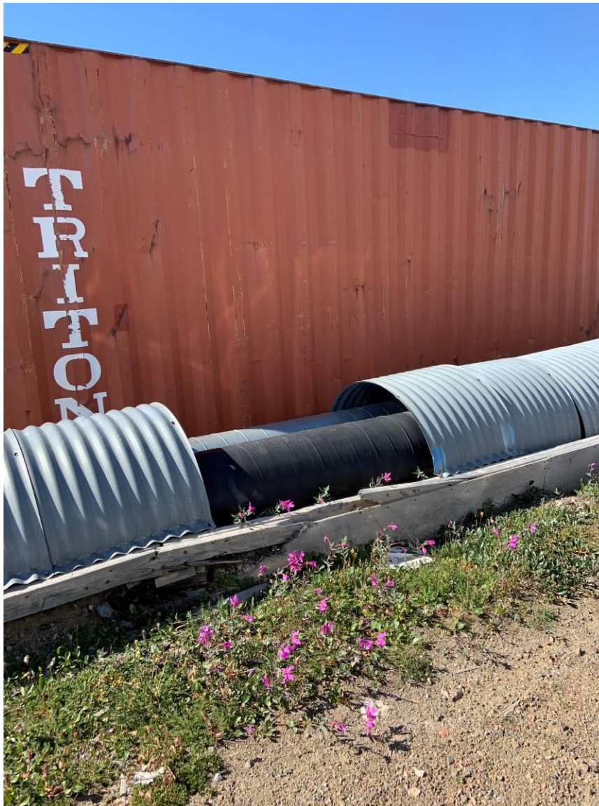
Photograph 9 – Section of the supply pipe from the dam with the corrugates metal enclosure removed.
