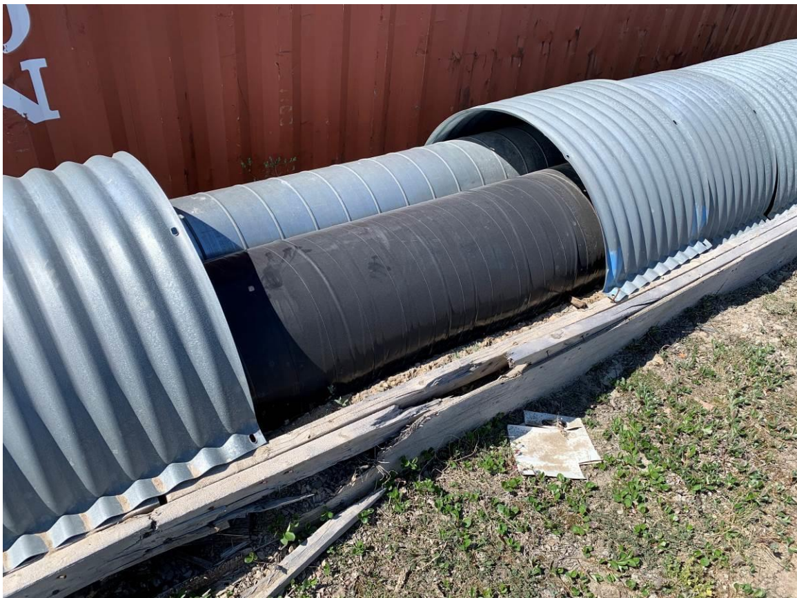
Photograph 13 – Section of the supply pipe from the dam with the corrugates metal enclosure removed.
