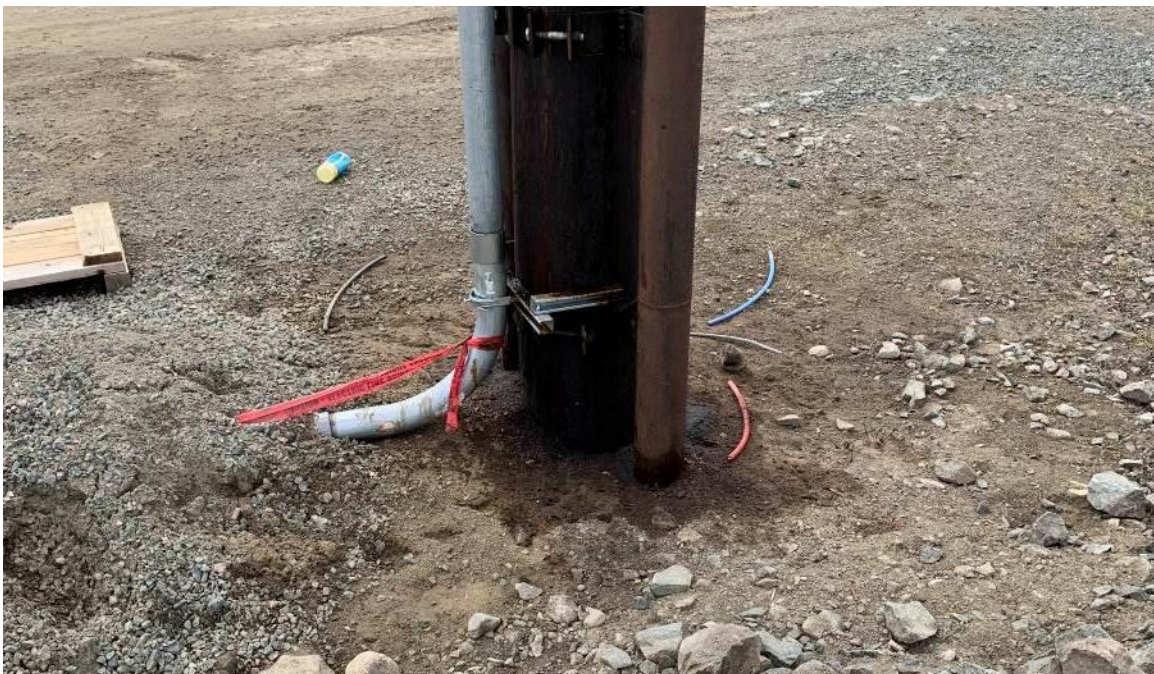
Photograph 5 – Oil residue on the ground around the base of the hydro pole, south berm.
