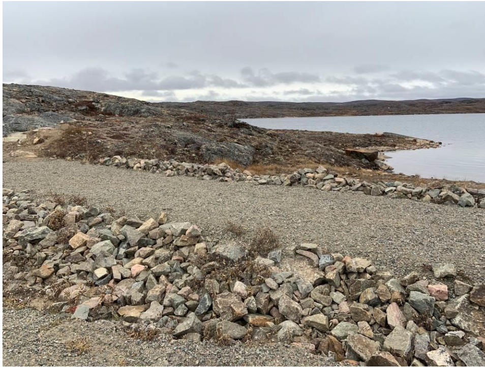
Photograph 12 – Displaced rip rap in South Berm.
