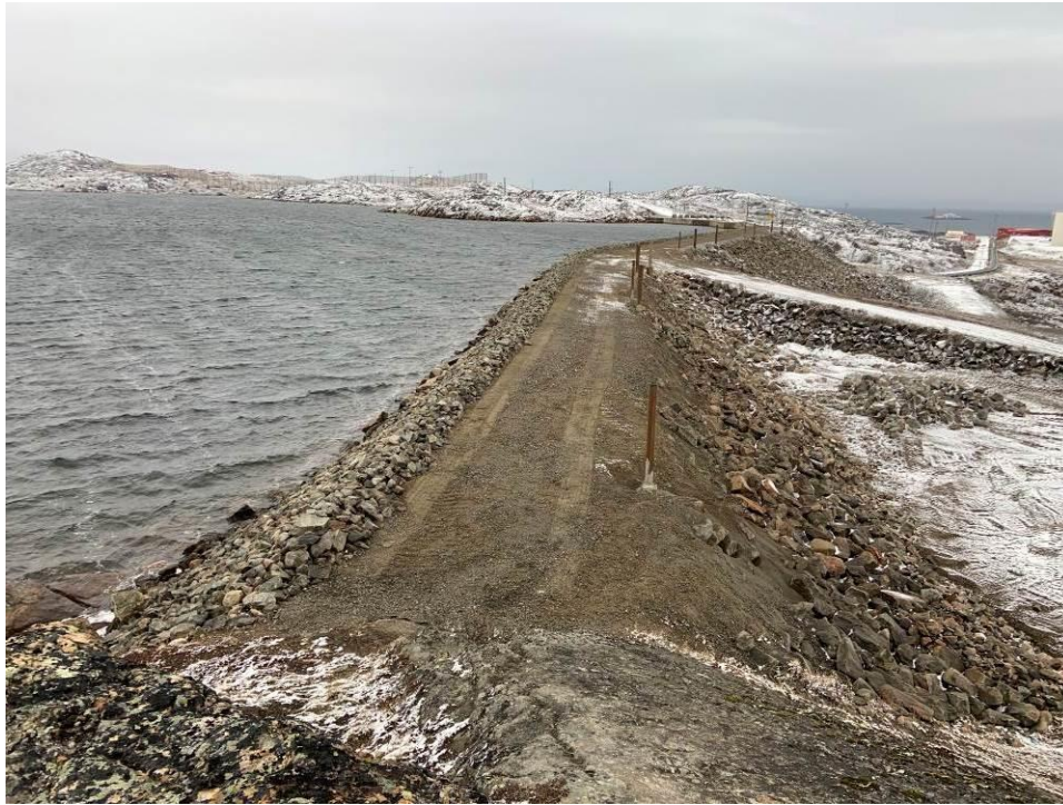
Photograph 3 – Typical north and center berm condition at the time of our review. New monitoring stations installed.
