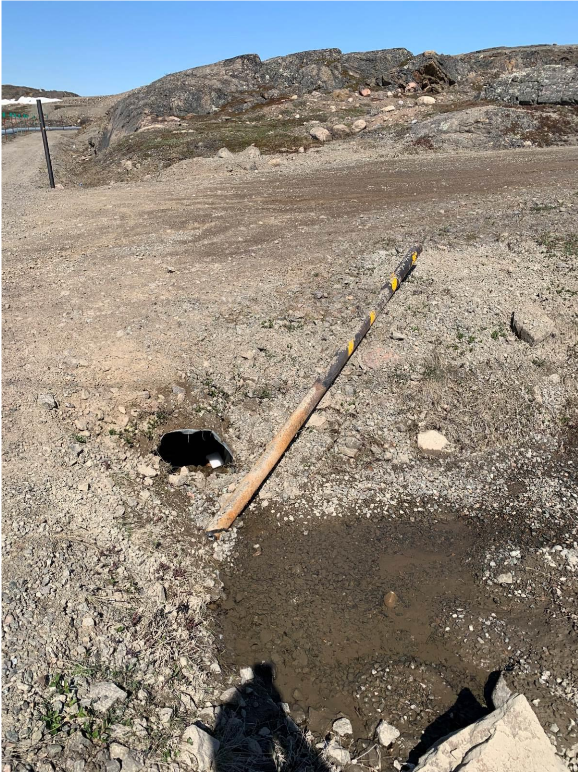
Photograph 11 – Corner marker at the junction of the south access road and the road to the south berm has been knocked over.
