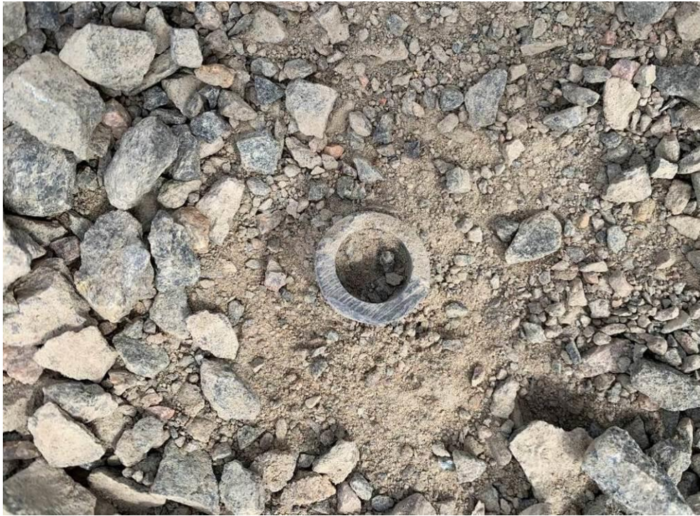
Photograph 7 – Borehole tube for piezometer blocked with aggregate material.
