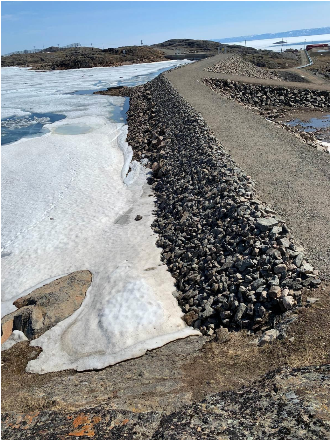
Photograph 3 – Typical north and center berm condition at the time of our review.
