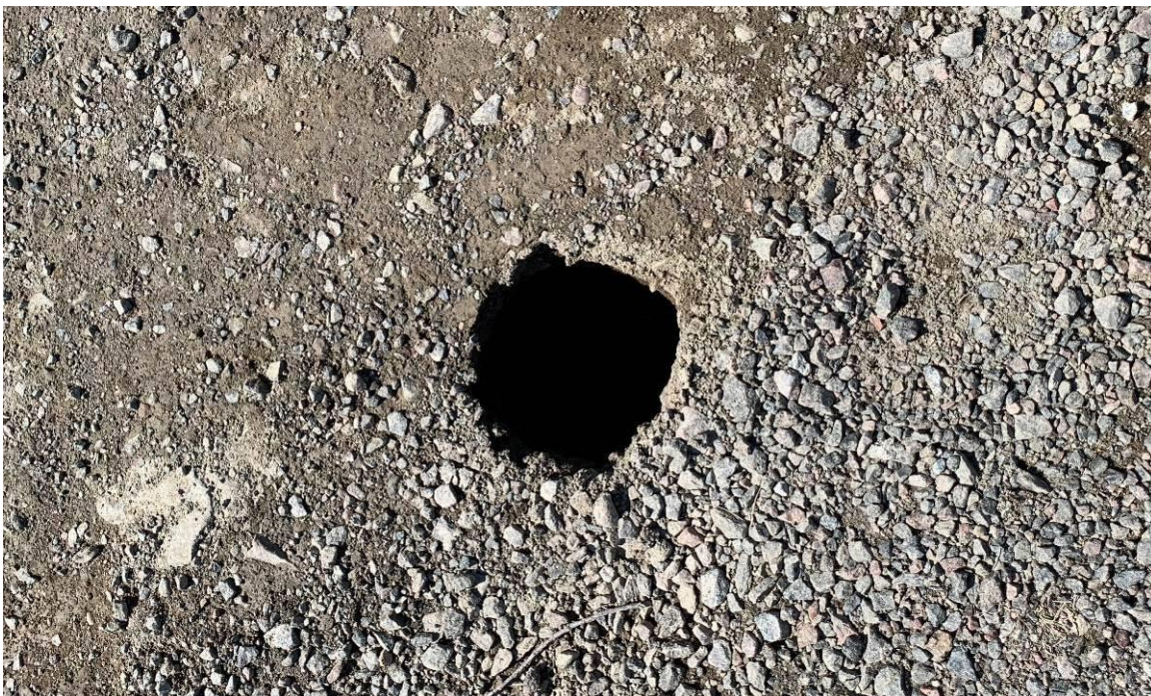
Photograph 7 –Sink hole within the south access road, approximately 40' south of the access gate.
