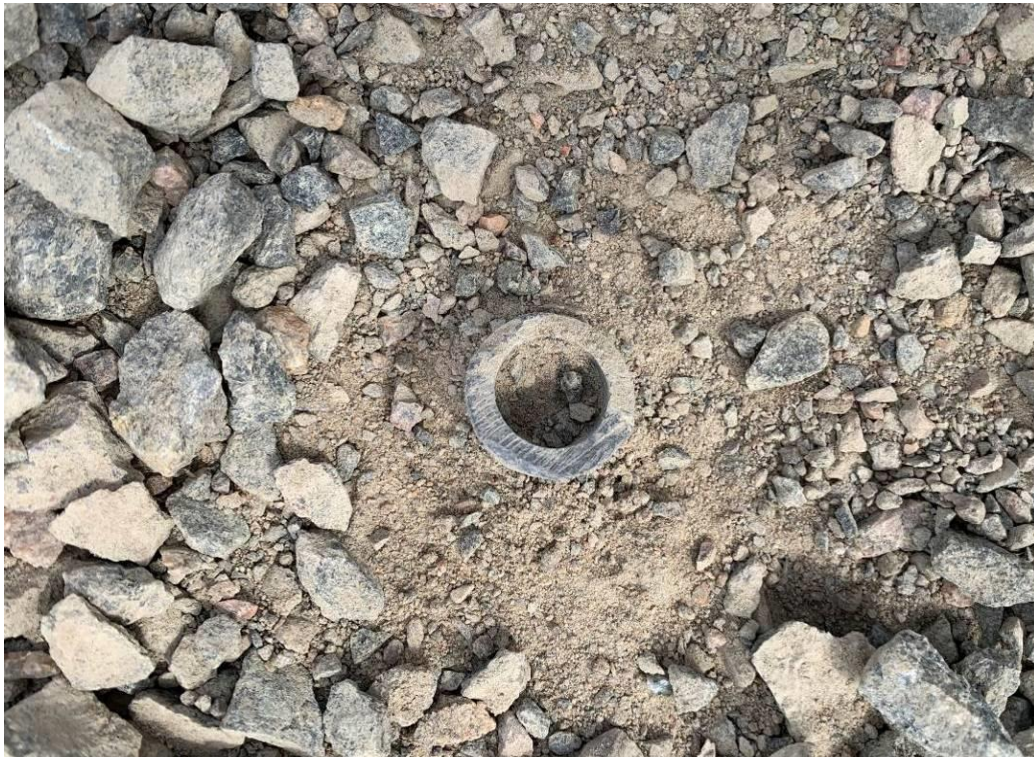
Photograph 10 – Borehole tube for piezometer blocked with aggregate material.
