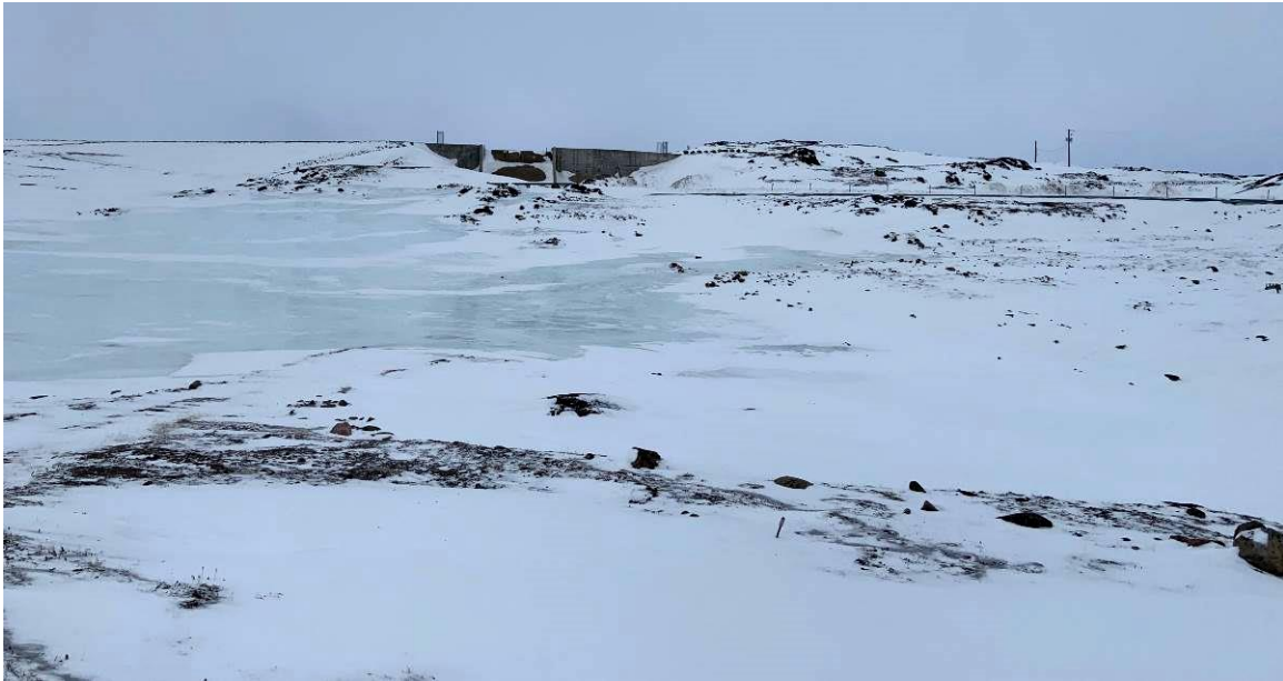
Photograph 5 – Snow and ice accumulation within the valley downstream of the concrete dam and earthen berms.
