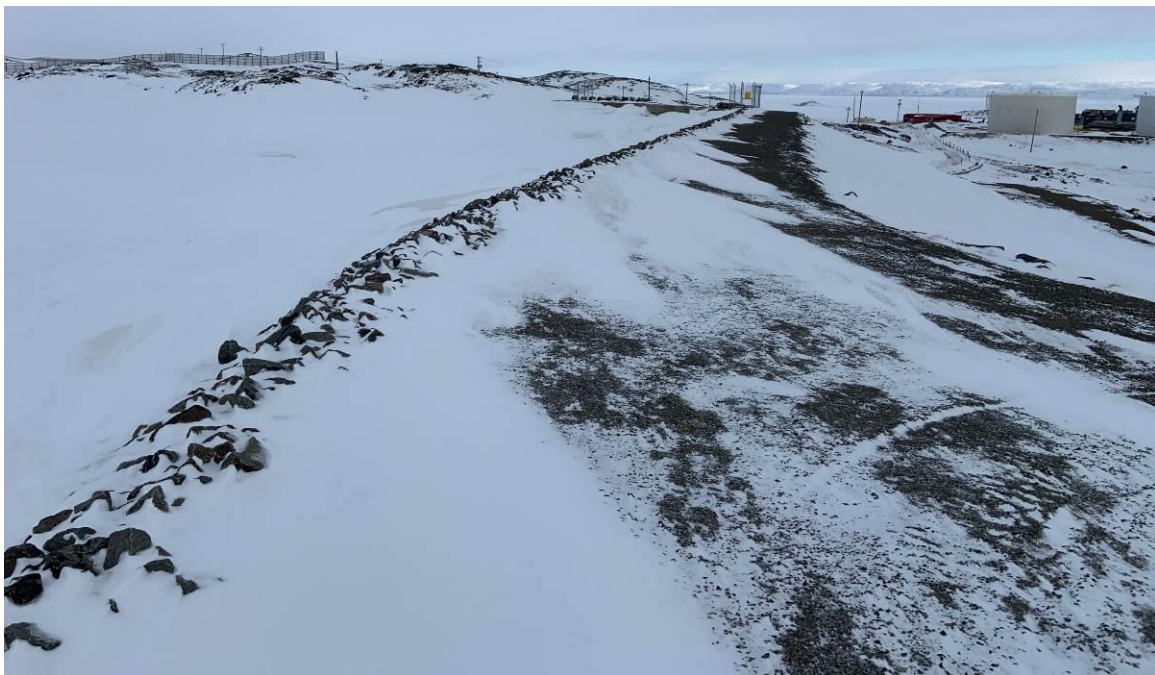
Photograph 2 – Typical center berm condition at the time of our review.
