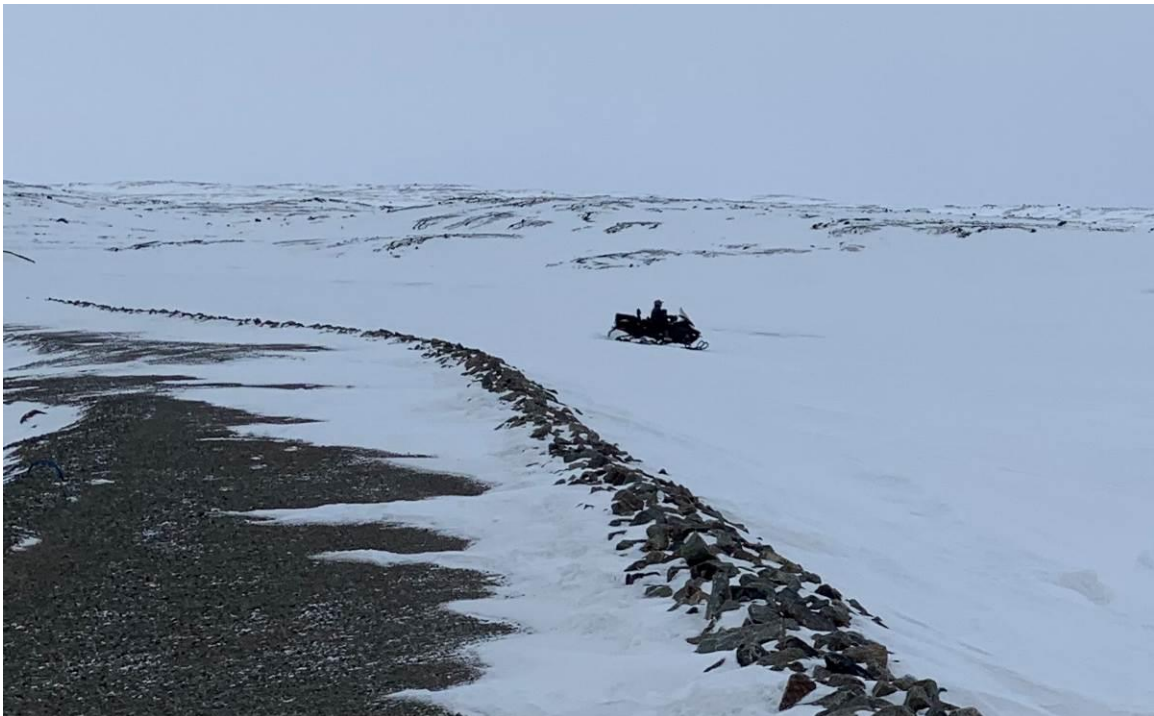
Photograph 6 – Typical public access atop and over the dam and onto the reservoir.
