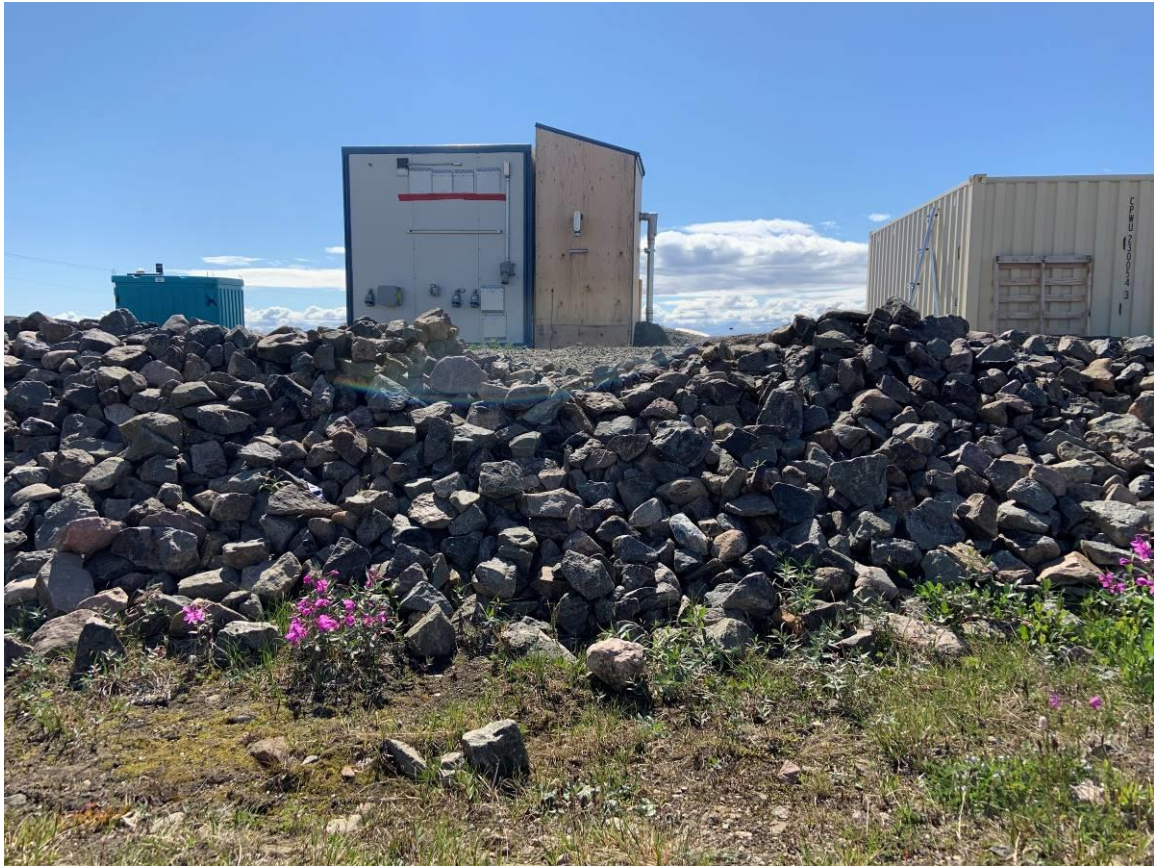
Photograph 12 – Displaced rip rap in South Berm
