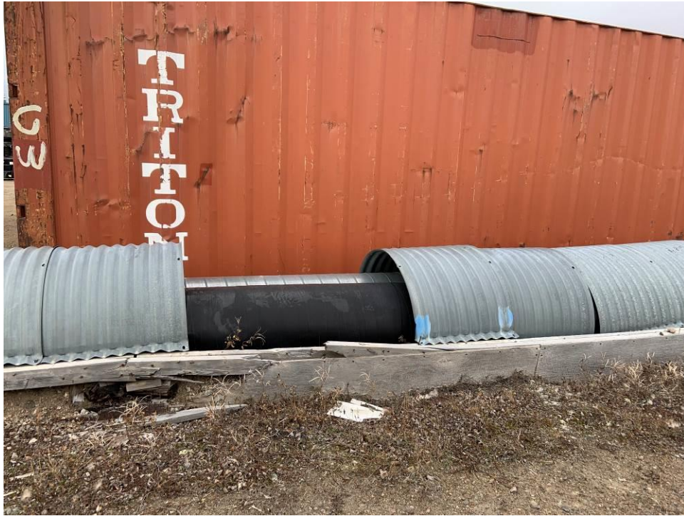
Photograph 9 – Section of the supply pipe from the dam with the corrugates metal enclosure removed.
