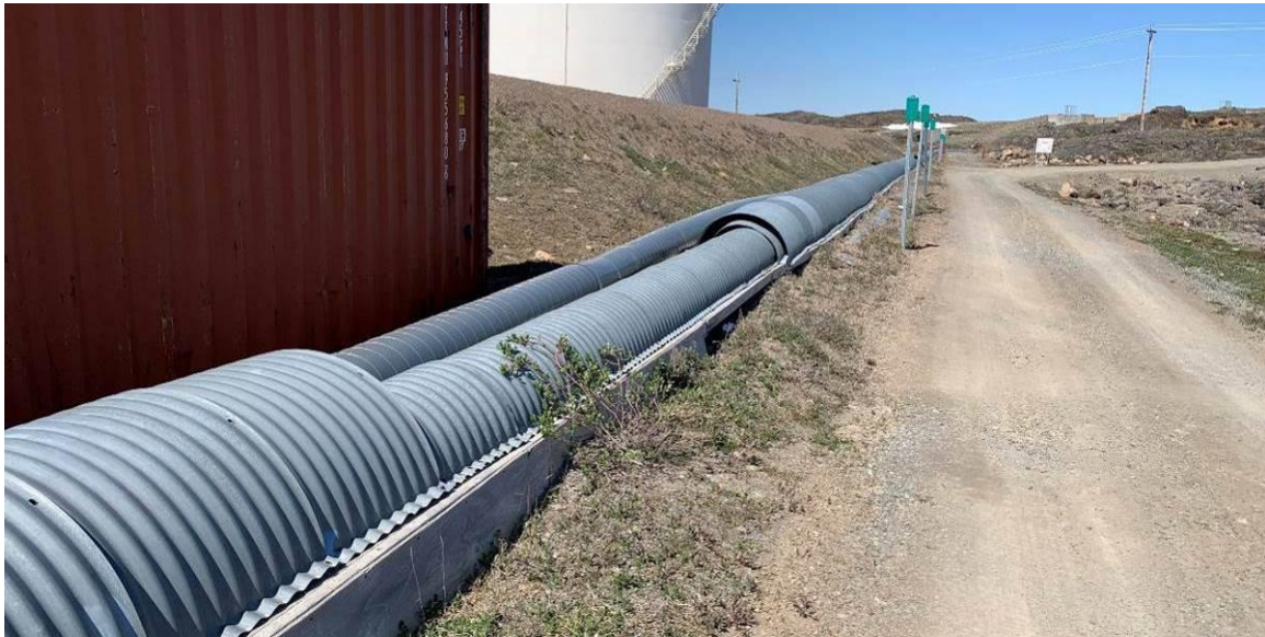
Photograph 12 – Section of the supply pipe from the dam with the corrugates metal enclosure removed.
