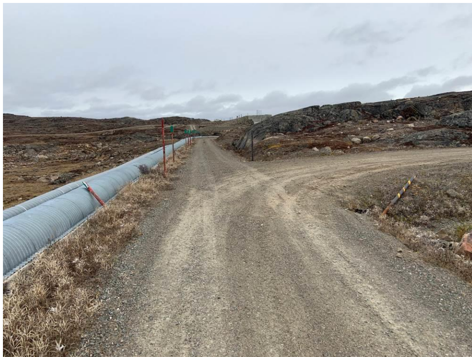
Photograph 8 – Corner marker at the junction of the south access road and the road to the south berm has been knocked over.
