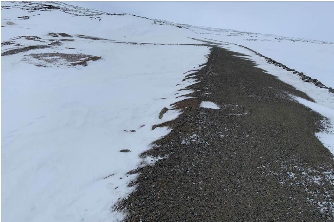
Photograph 4 – Typical snow and ice accumulation on the downstream face of the north and center berms.
