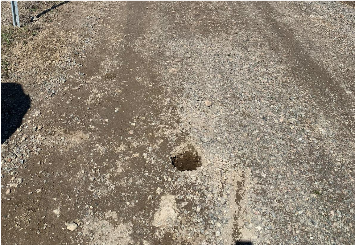
Photograph 6 –Sink hole within the south access road, approximately 40' south of the access gate.
