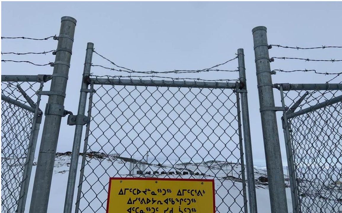
Photograph 7 – Typical damage to the fencing atop the dam.
