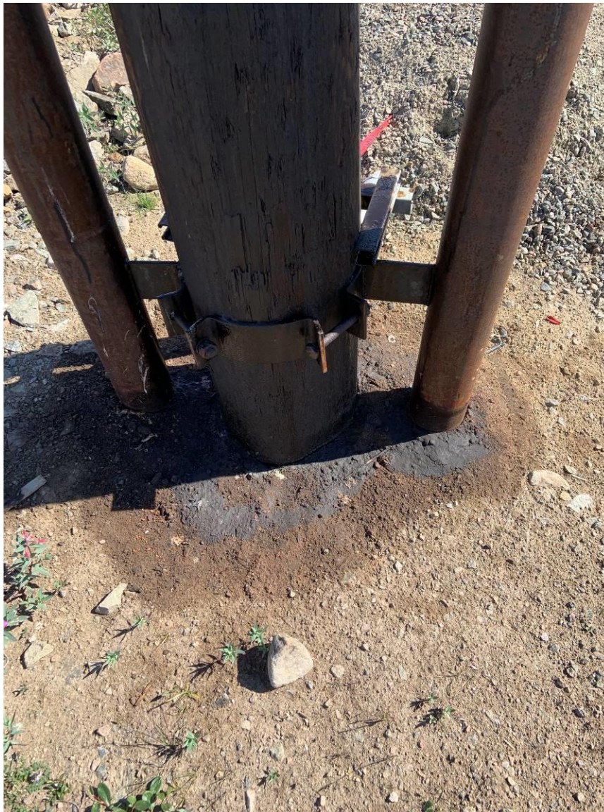
Photograph 4 – Oil residue on the ground around the base of the hydro pole, south berm.
