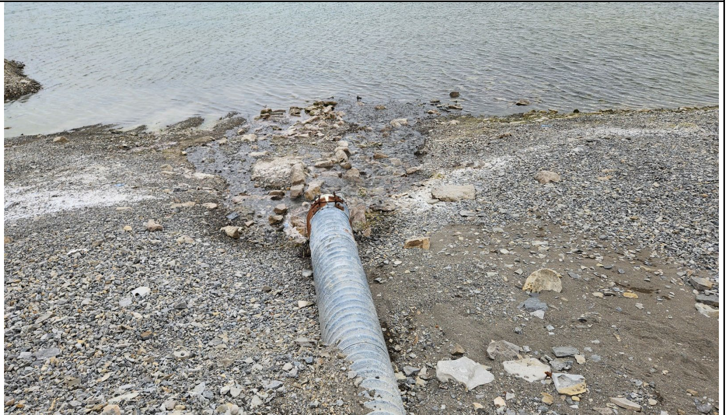
Description: Utilidor Sewage Discharge Pipe. Direct Discharge to the ocean.
