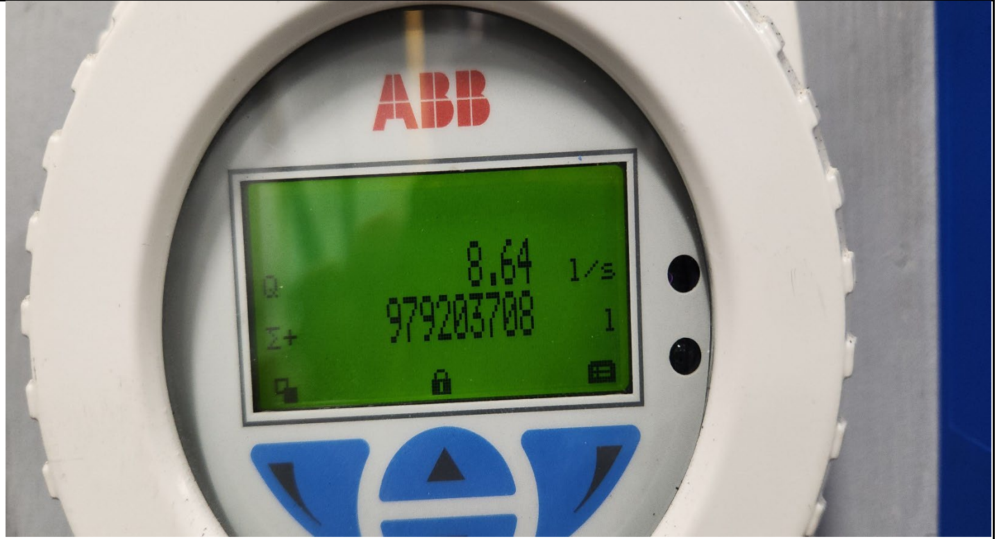
Description: ABB meter observed in the water pump house. 979203708Litres, 979203.708 m 3
