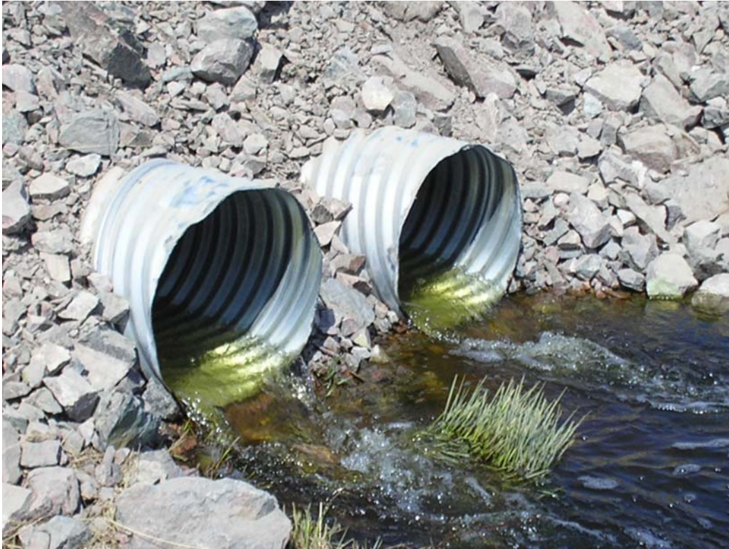
Figure 19: Water discharging into Airplane Lake through culvert under road.
