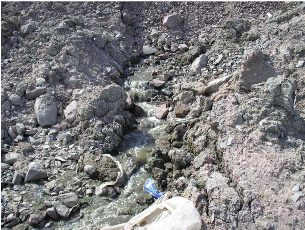
Figure 4: Water leaking out the base of the berm at the center of the north side of the berm.
