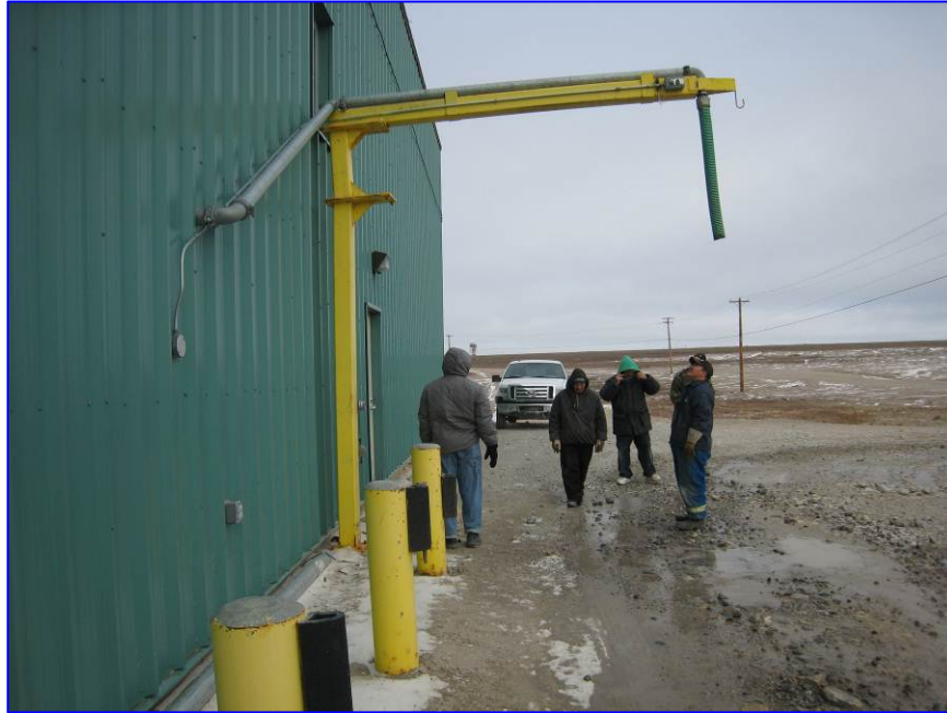
Photograph No. 21 Truck fill station.
