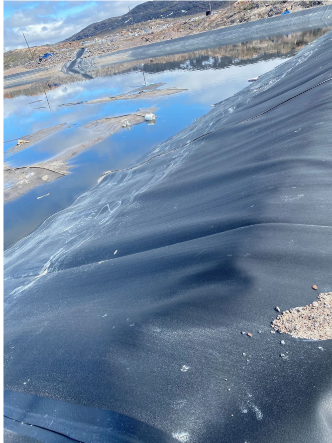
2023 Liner Bubbles - West Side south of vent
