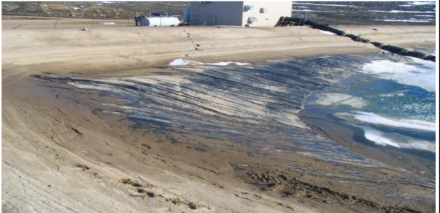
Water Intake Pipe - Reservoir
