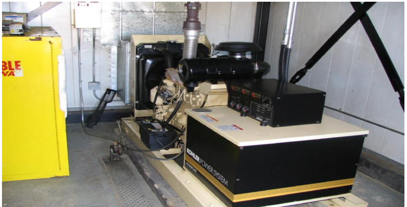
Diesel Generator (1 of 2)
