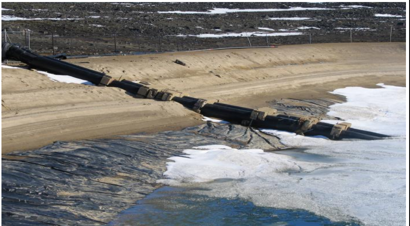
Water Intake Pipe - Reservoir
