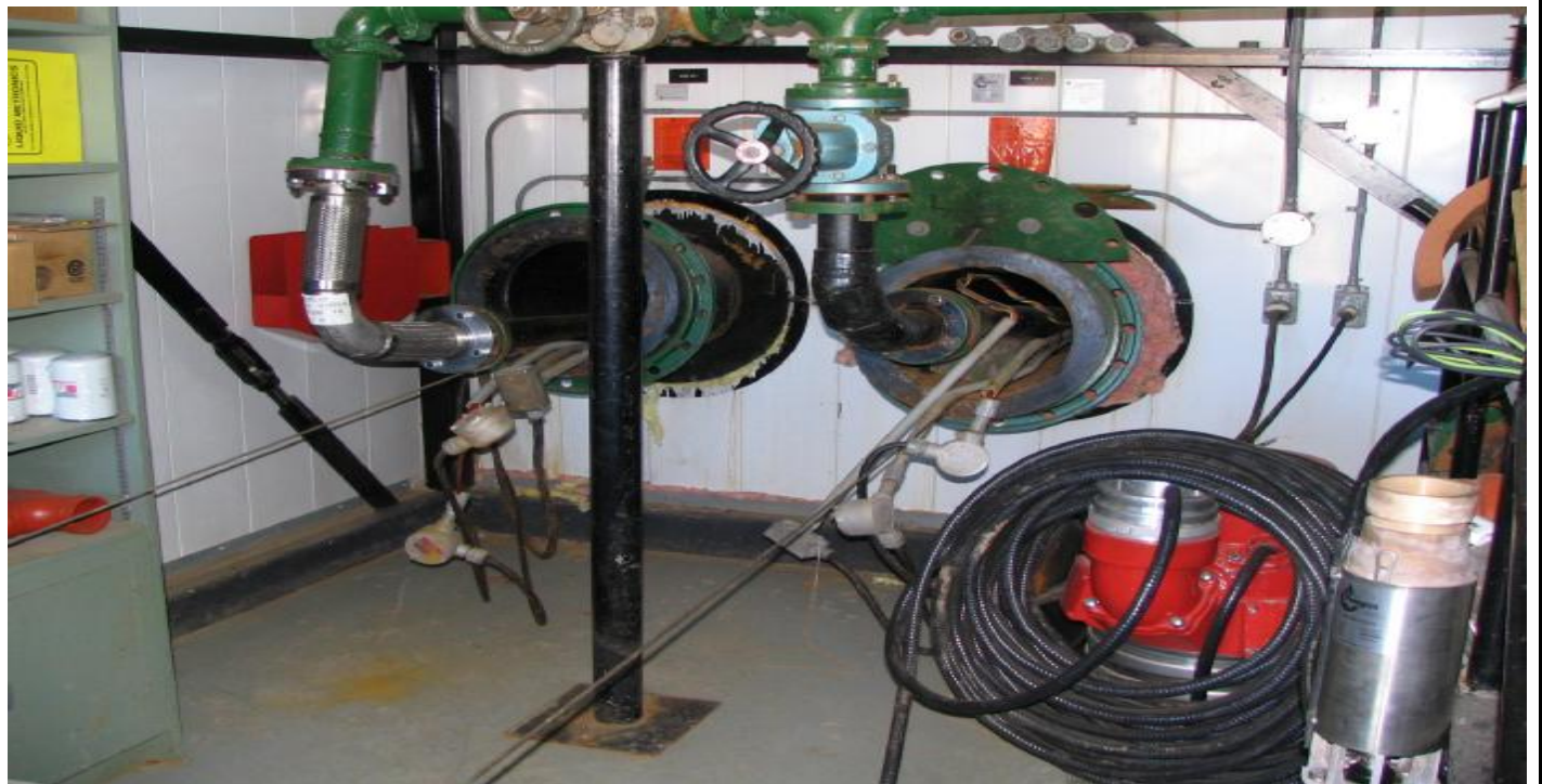
Intake Pipe Entering Existing Pumphouse
