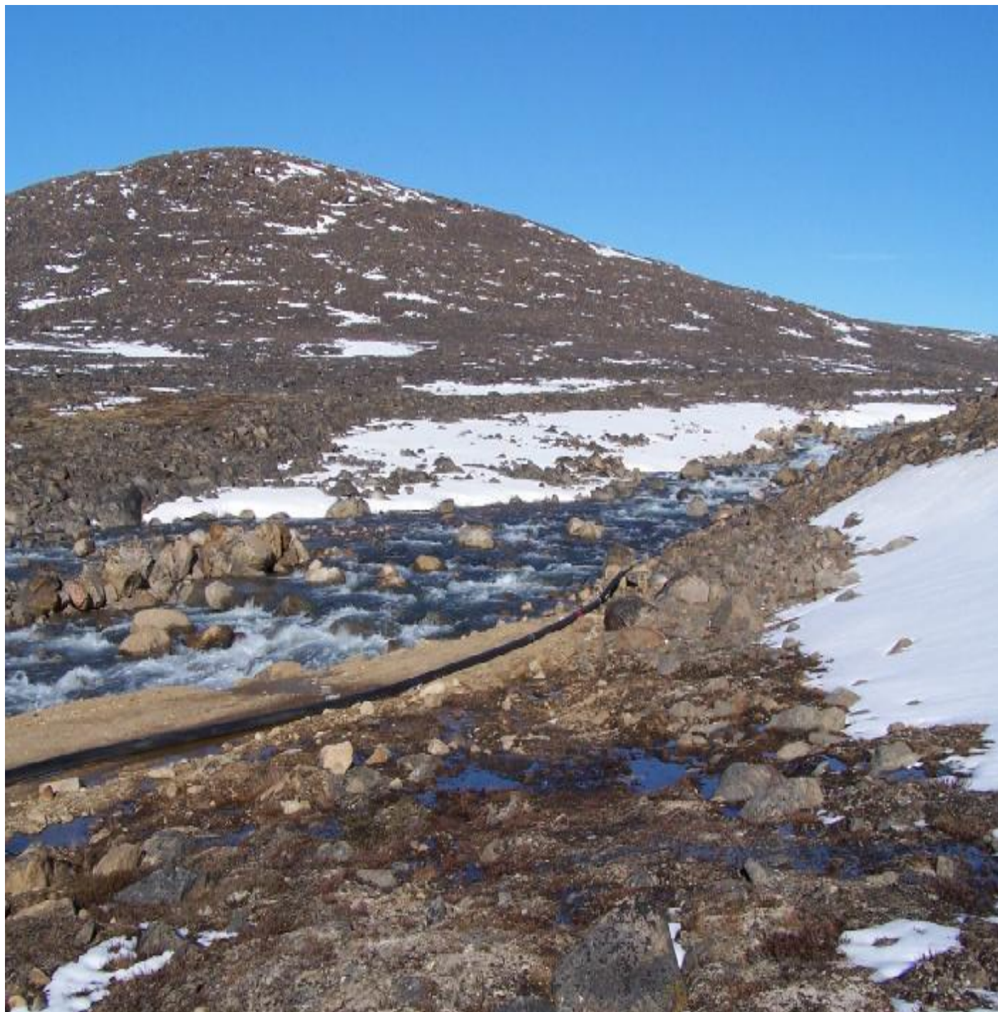
Raw Water Intake Pipe
