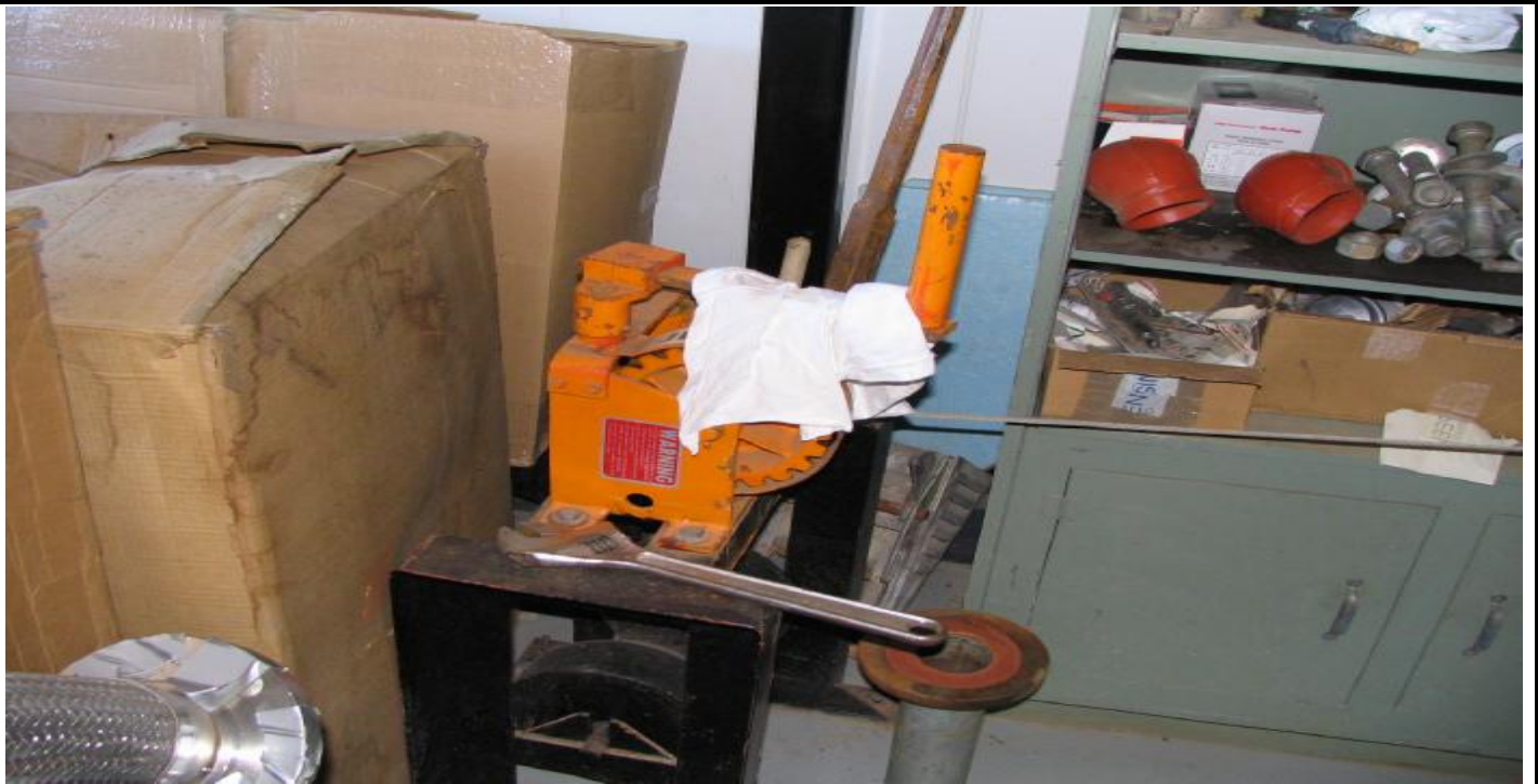
Winch for Reservoir Pump Removal
