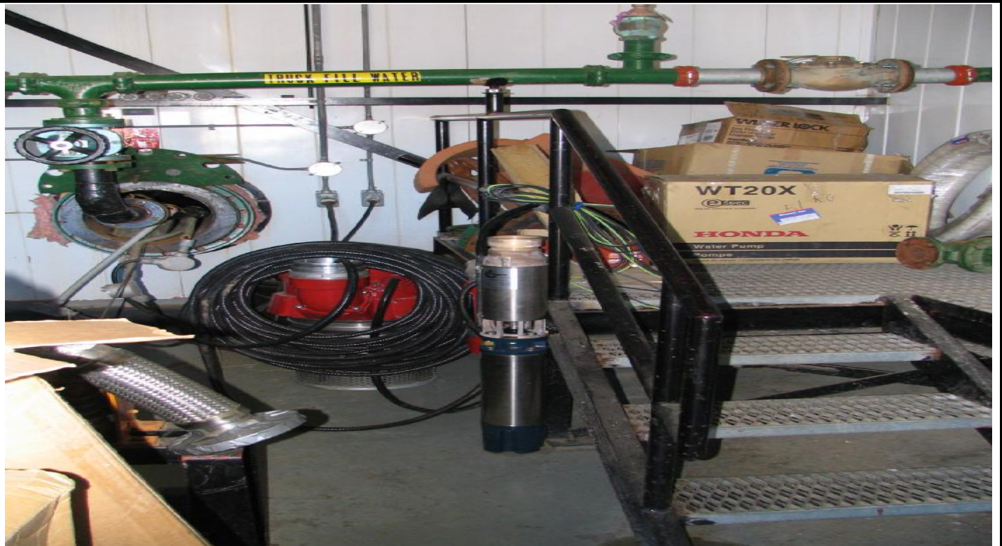
Truck fill Piping within existing Pumphouse
