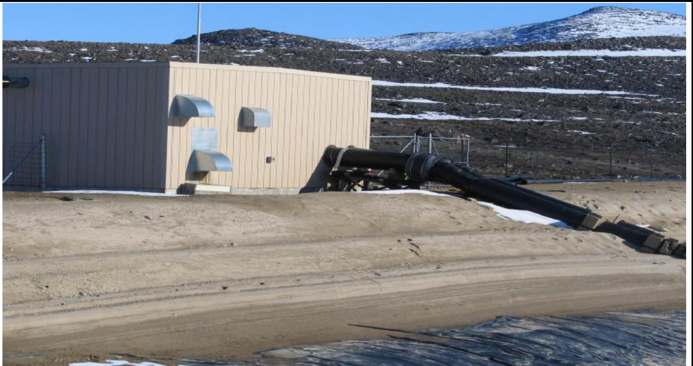
Water Intake Pipe - Reservoir
