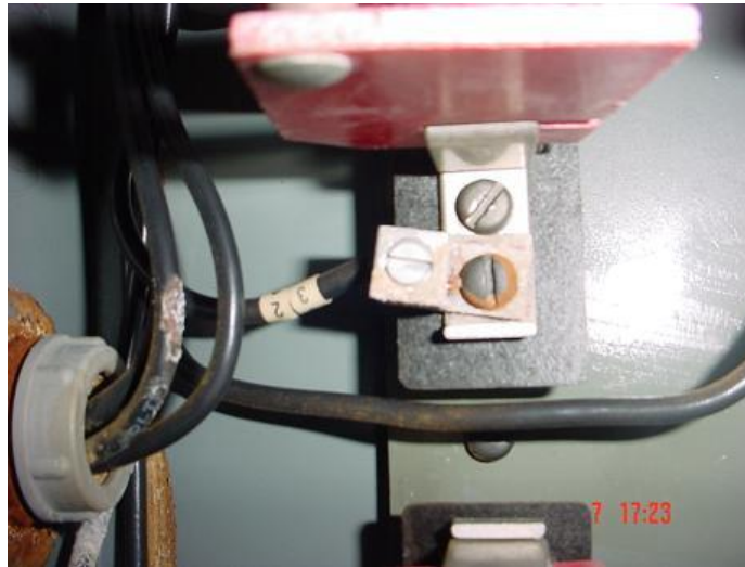
Figure E-17: Dust Build-Up on Lugs
