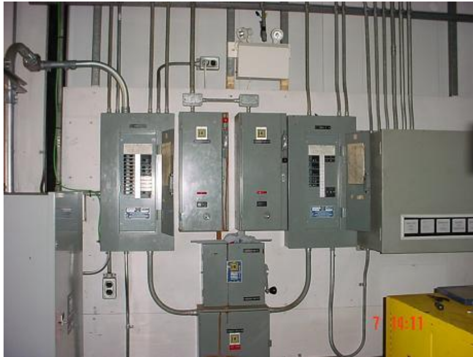
Figure E-4: Distribution Panels
