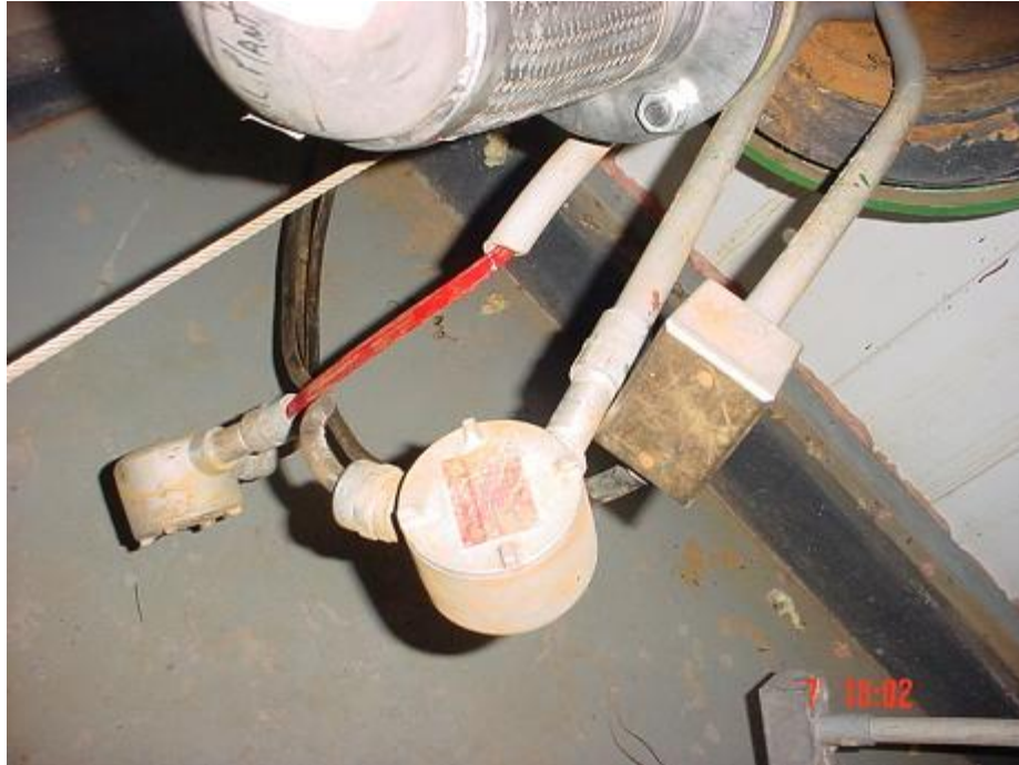
Figure E-11: Broken PVC Fittings
