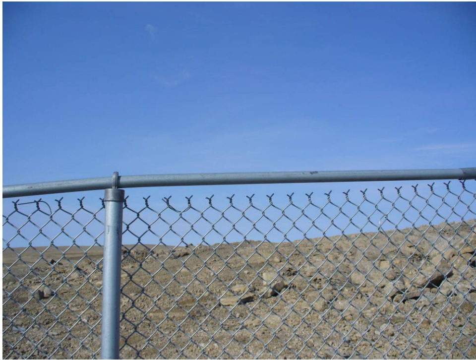
Figure 40: Chain link short from top rail.
