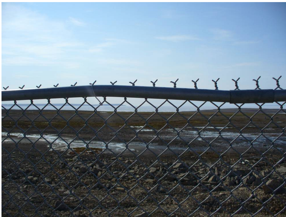
Figure 37: Localized bent top rail.
