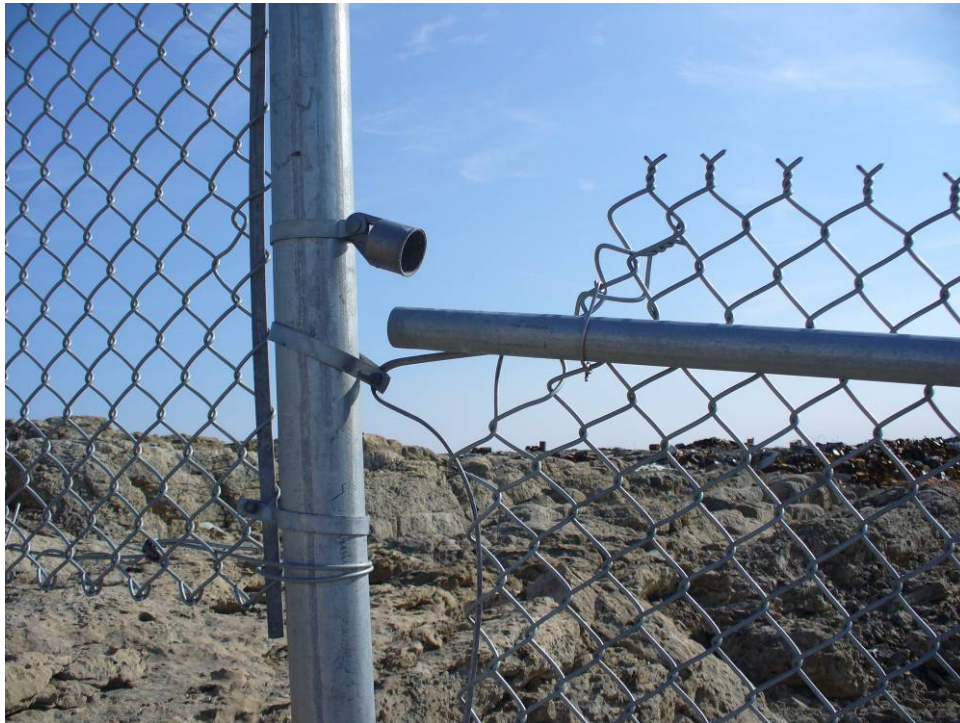
Figure 36: Top rail connection, disconnected.
