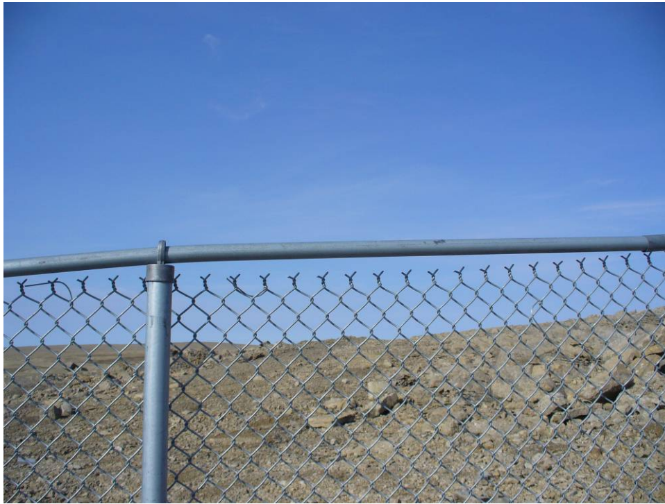
Figure 40: Chain link short from top rail.
