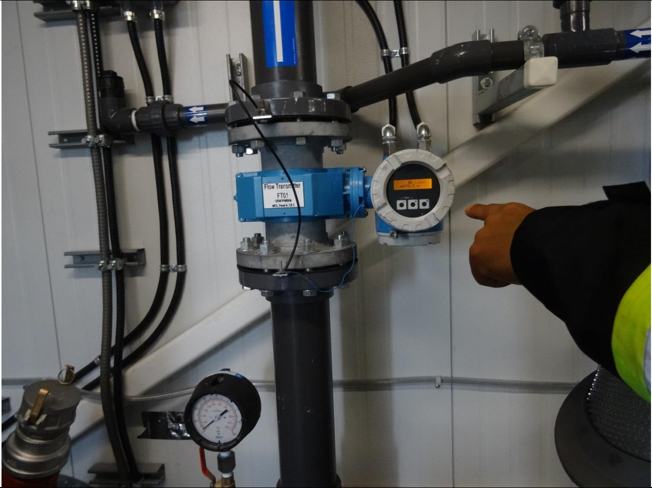
Description: Raw Water Intake Flow Meter used by the Hamlet to Calculate/Record overall Consumption amounts
