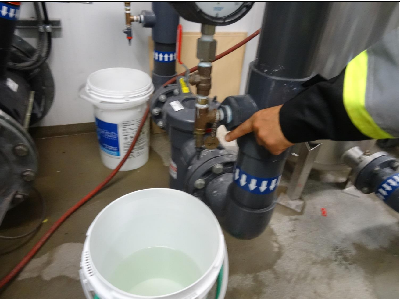
Description: TAL-1 Indoor Sample Area inside Water Treatment Plant – with Brass Tag Signage
