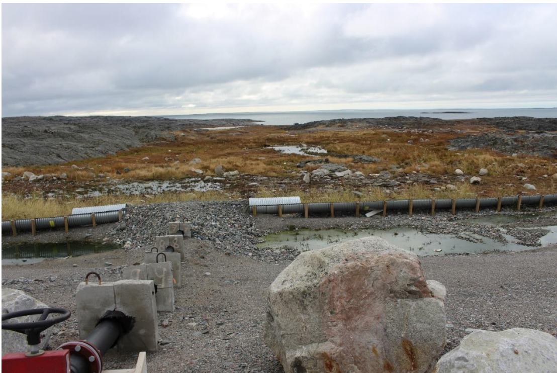
Figure 10 Discharge dispersion structure facing the wetland
