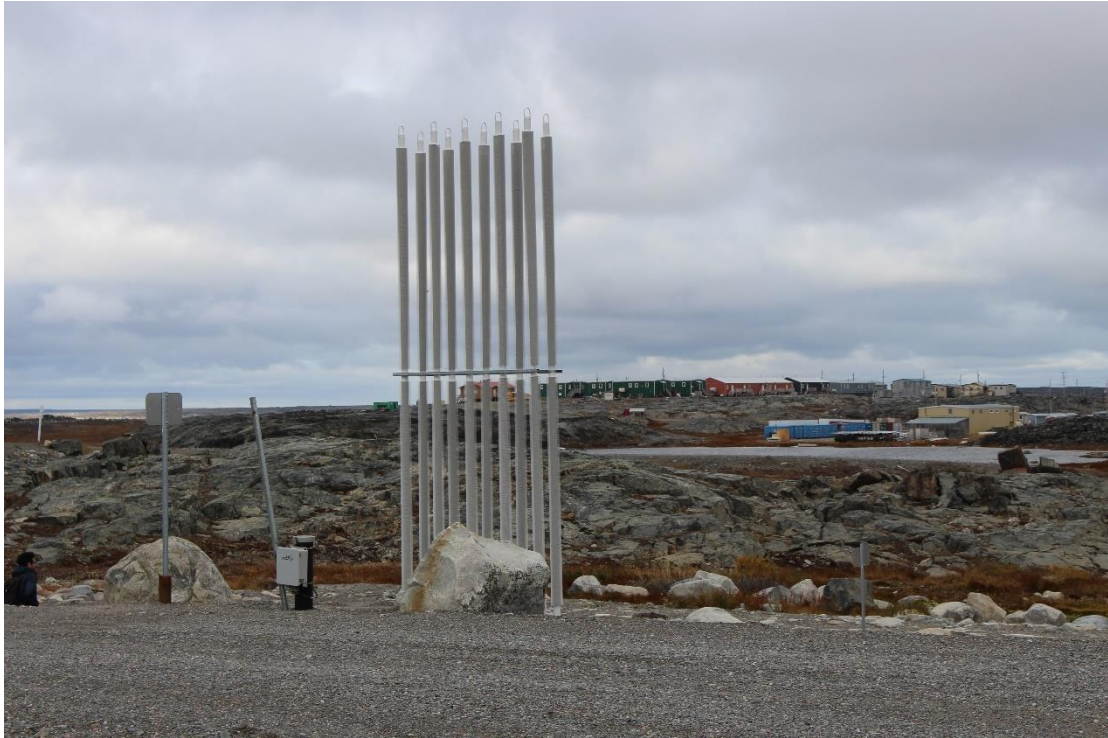
Figure 5 Radiators for the thermosiphons
