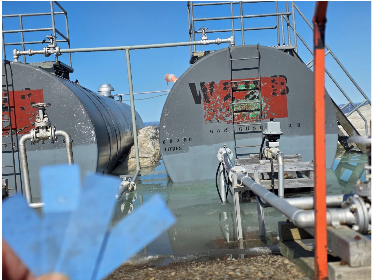
Photo E 1: Hydrocarbon test strips used in berm of tanks W22A & W22B (25-Jun-2025)
