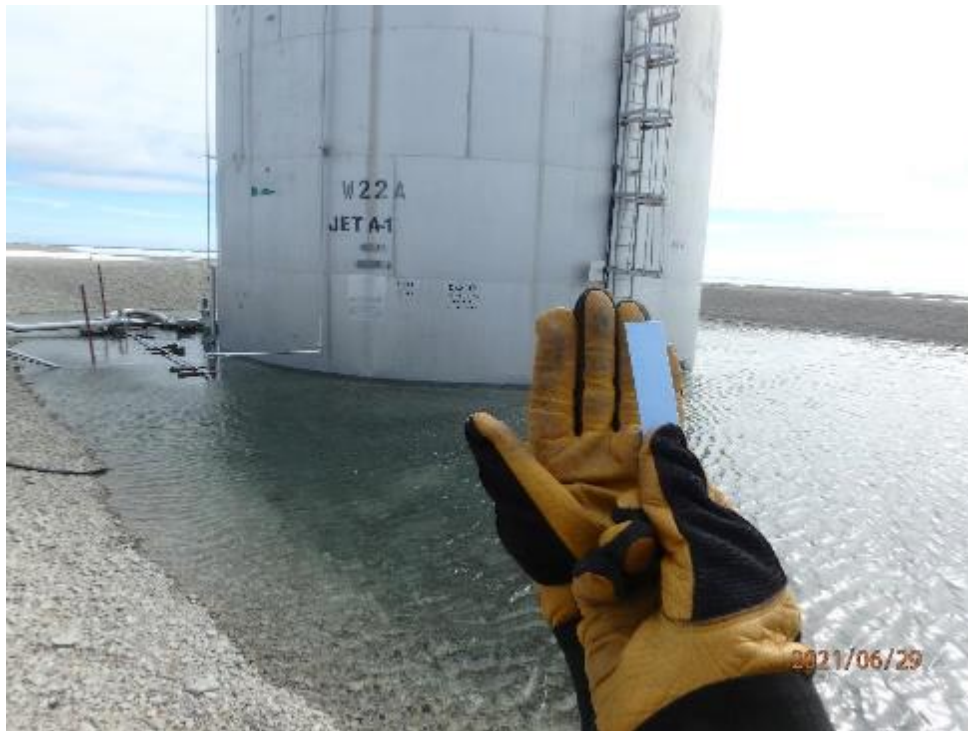
Photo E 8: Hydrocarbon test strips used in berm of tank W22A (29-Jun-2021)
