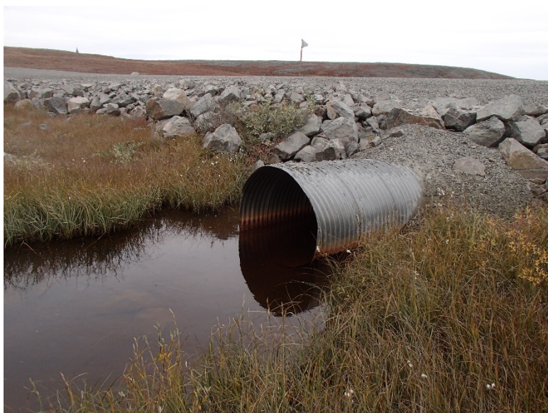
Photograph D1-32: R-05A km 15+745
