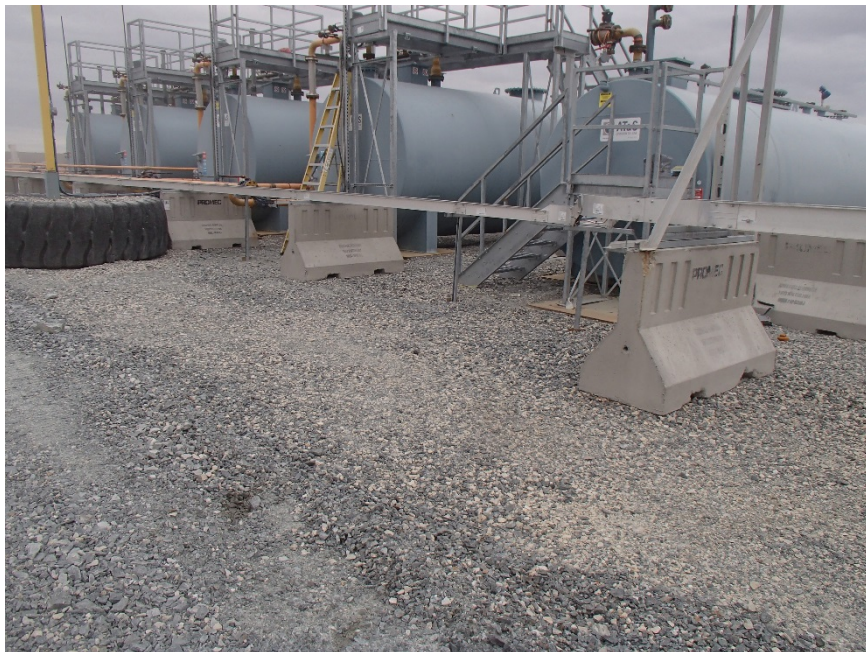
Photograph G3-1 Vault Tank Farm
