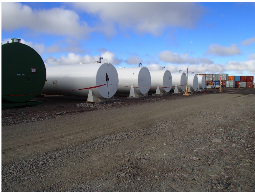
Photograph G4-2 Amaruq Tank Farm
