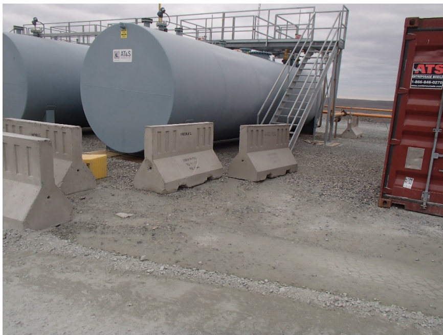
Photograph G3-2 Vault Tank Farm
