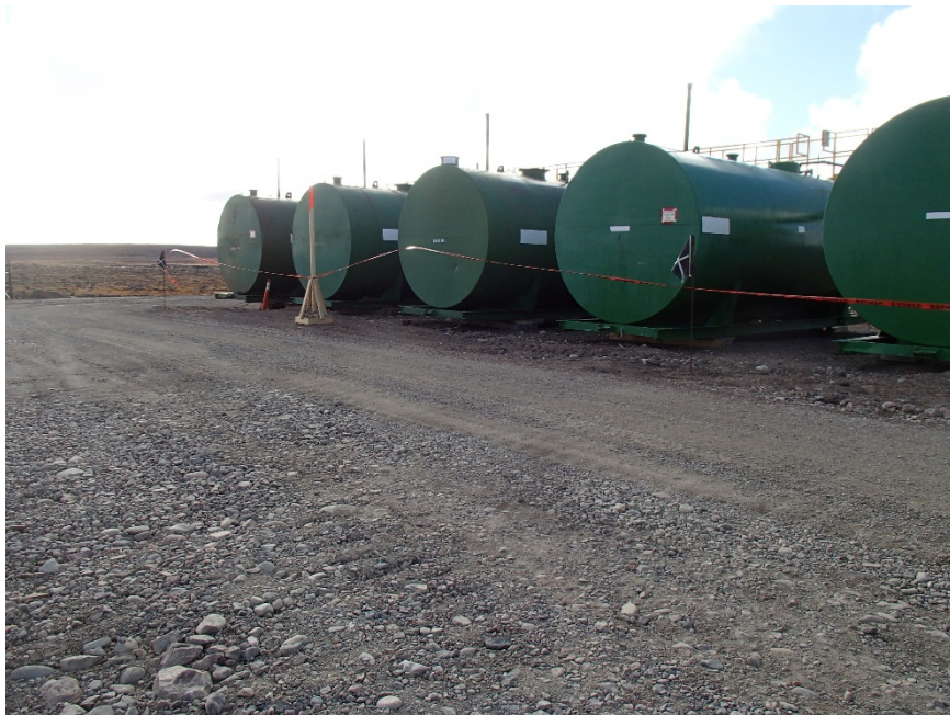
Photograph G4-1 Amaruq Tank Farm
