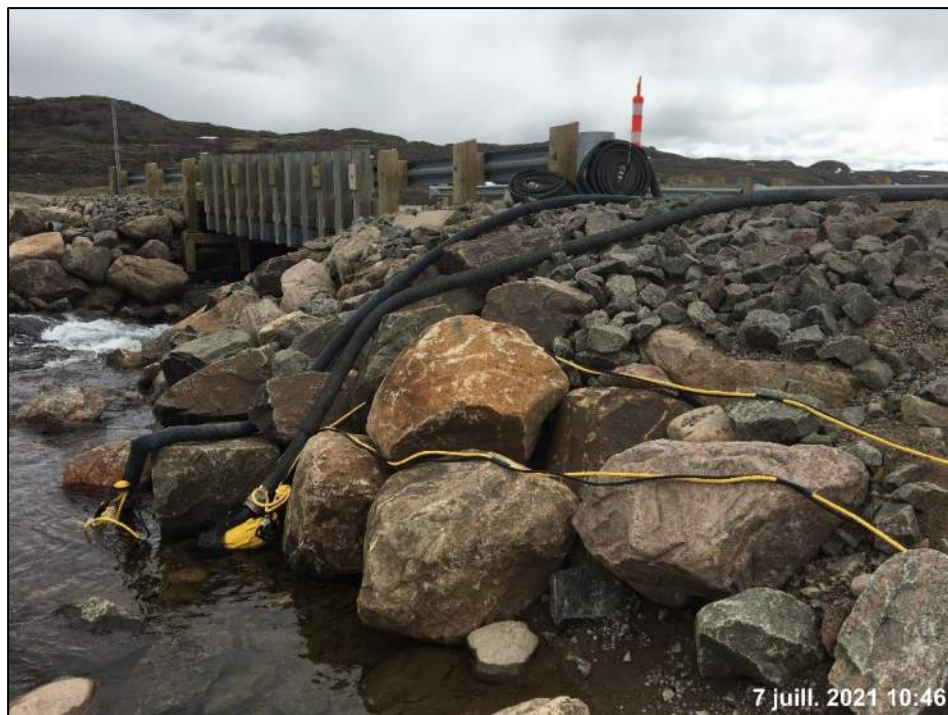
Pumps and hoses
