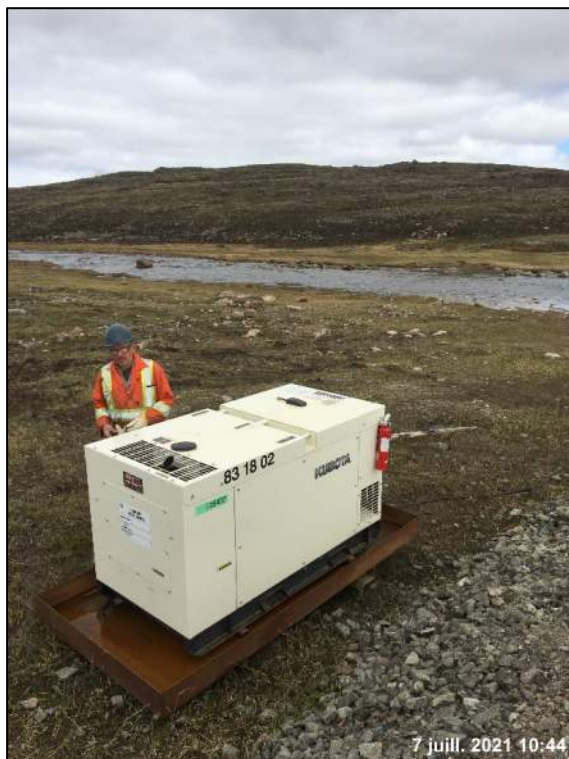
Generator with secondary containment
