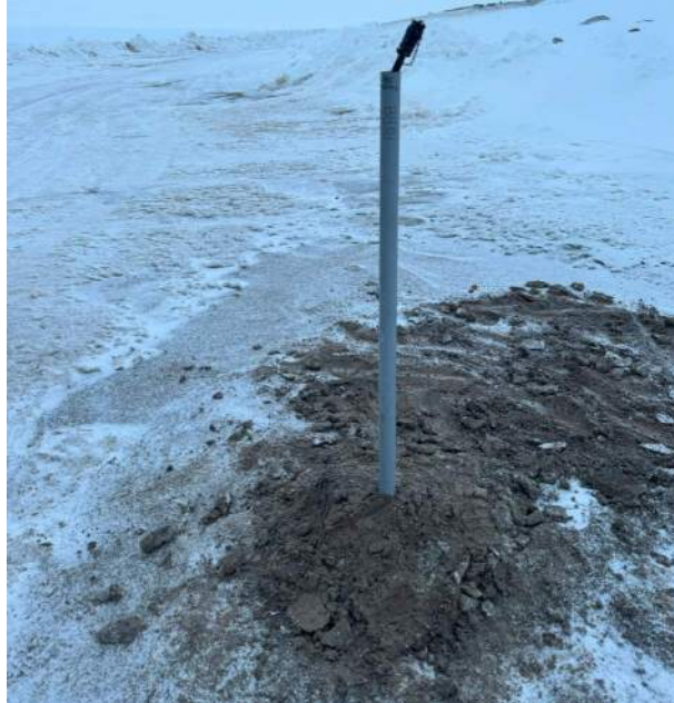
Photograph 7 Thermistor T1 installed in BH01.
