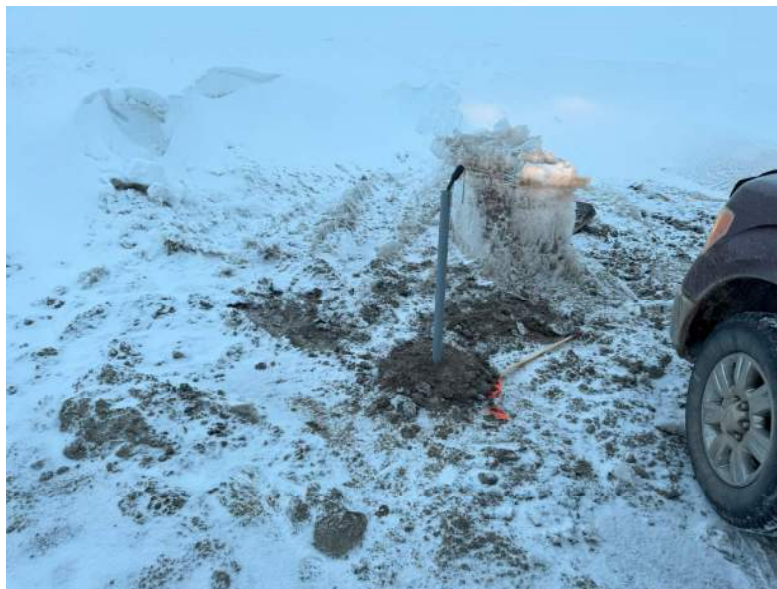
Photograph 8 Thermistor T2 installed in BH10.
